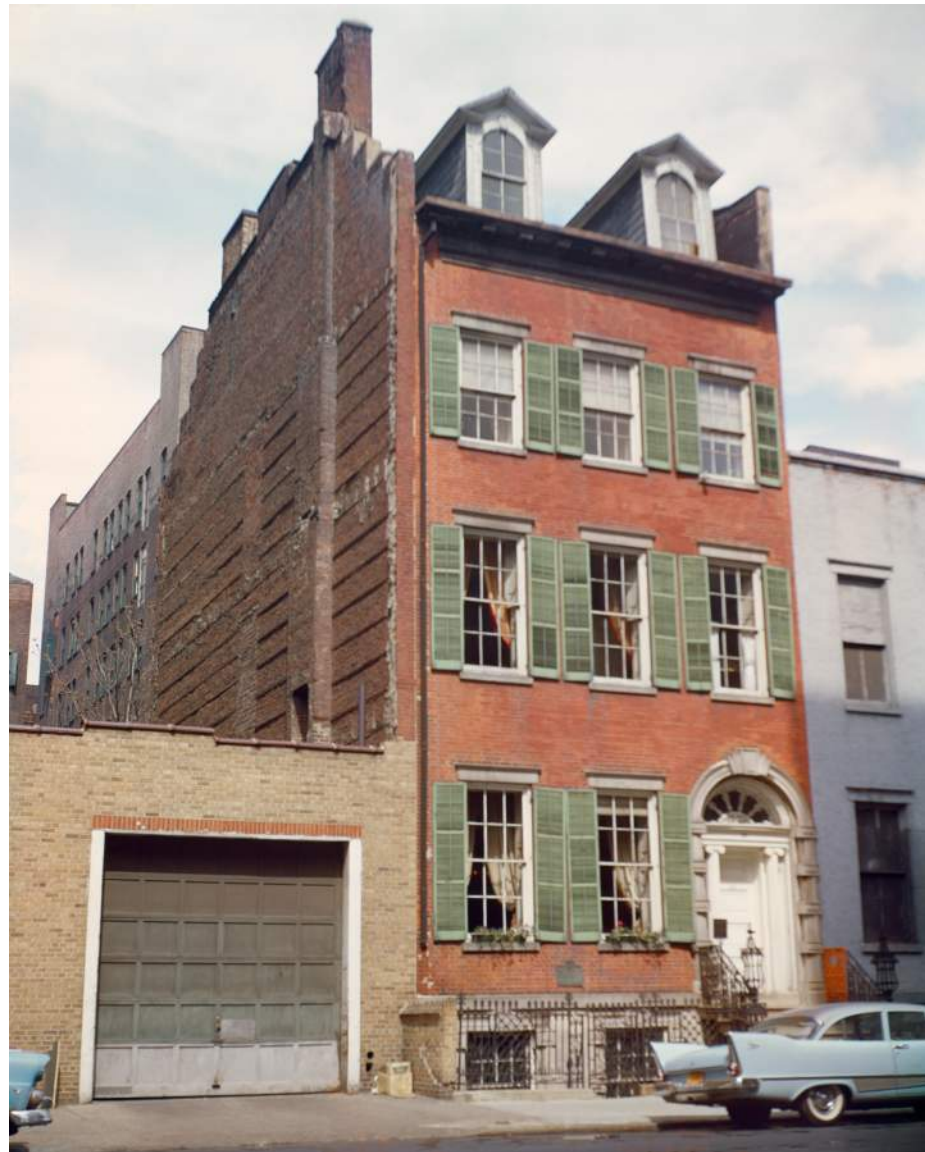
1960'S LOT LINE WALL CONDITION
