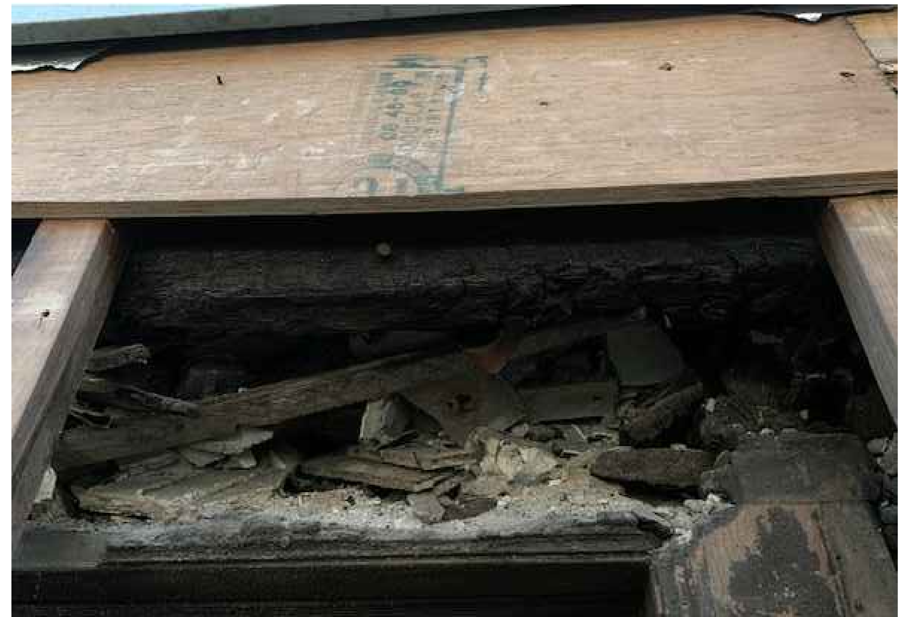
FACADE PROBE SHOWING FIRE DAMAGED FRAMING
