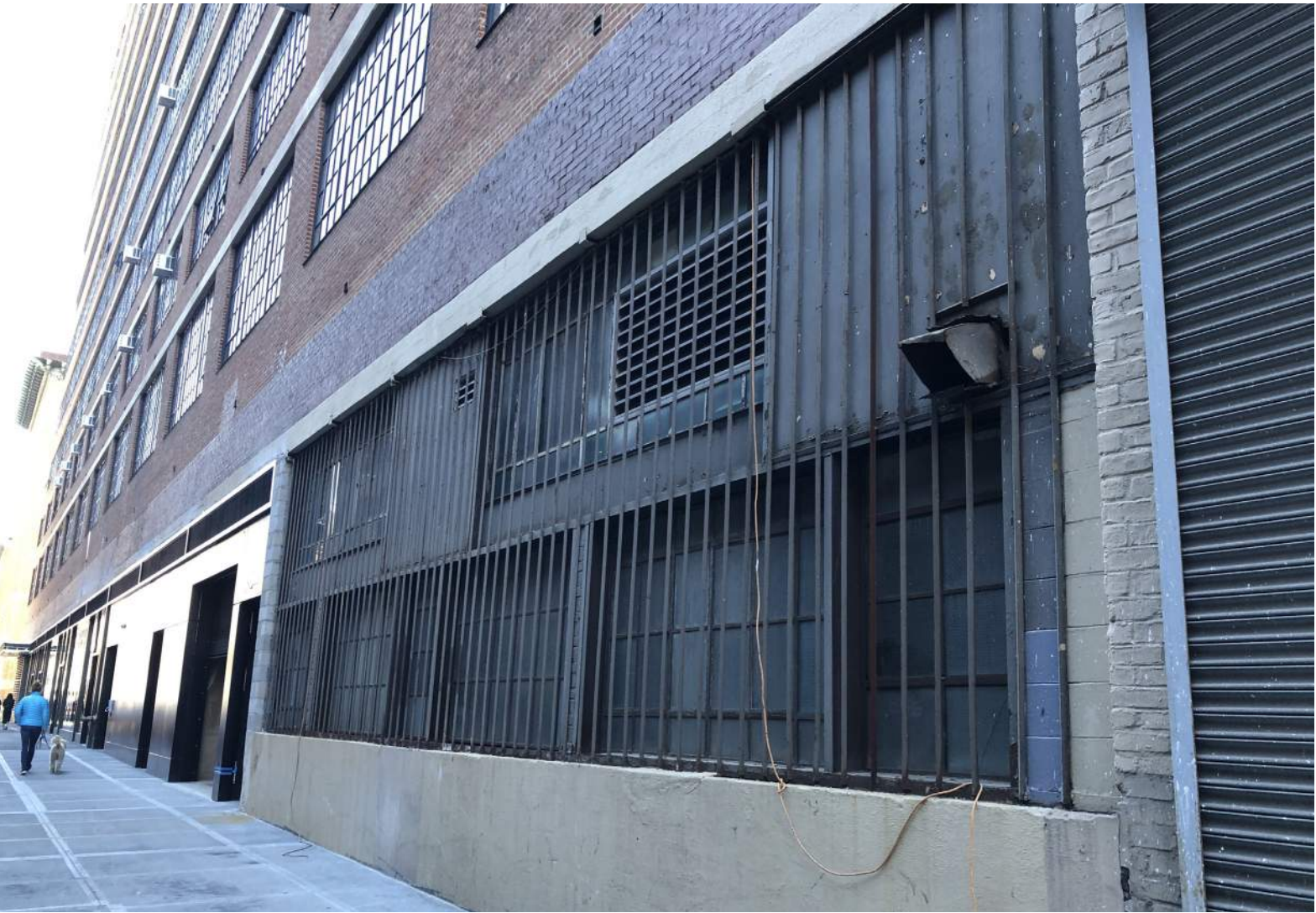
27th Street facade, frontal view at loading dock and proposed work location
