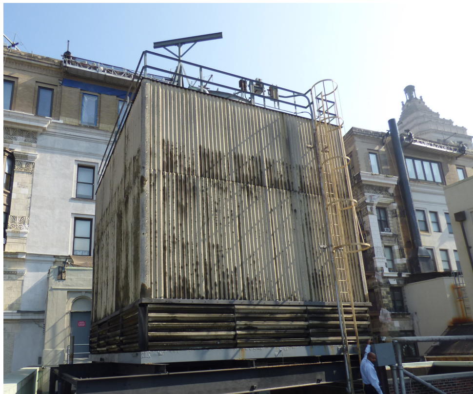
EXISTING COOLING TOWER AT WEST SIDE OF ROOF
