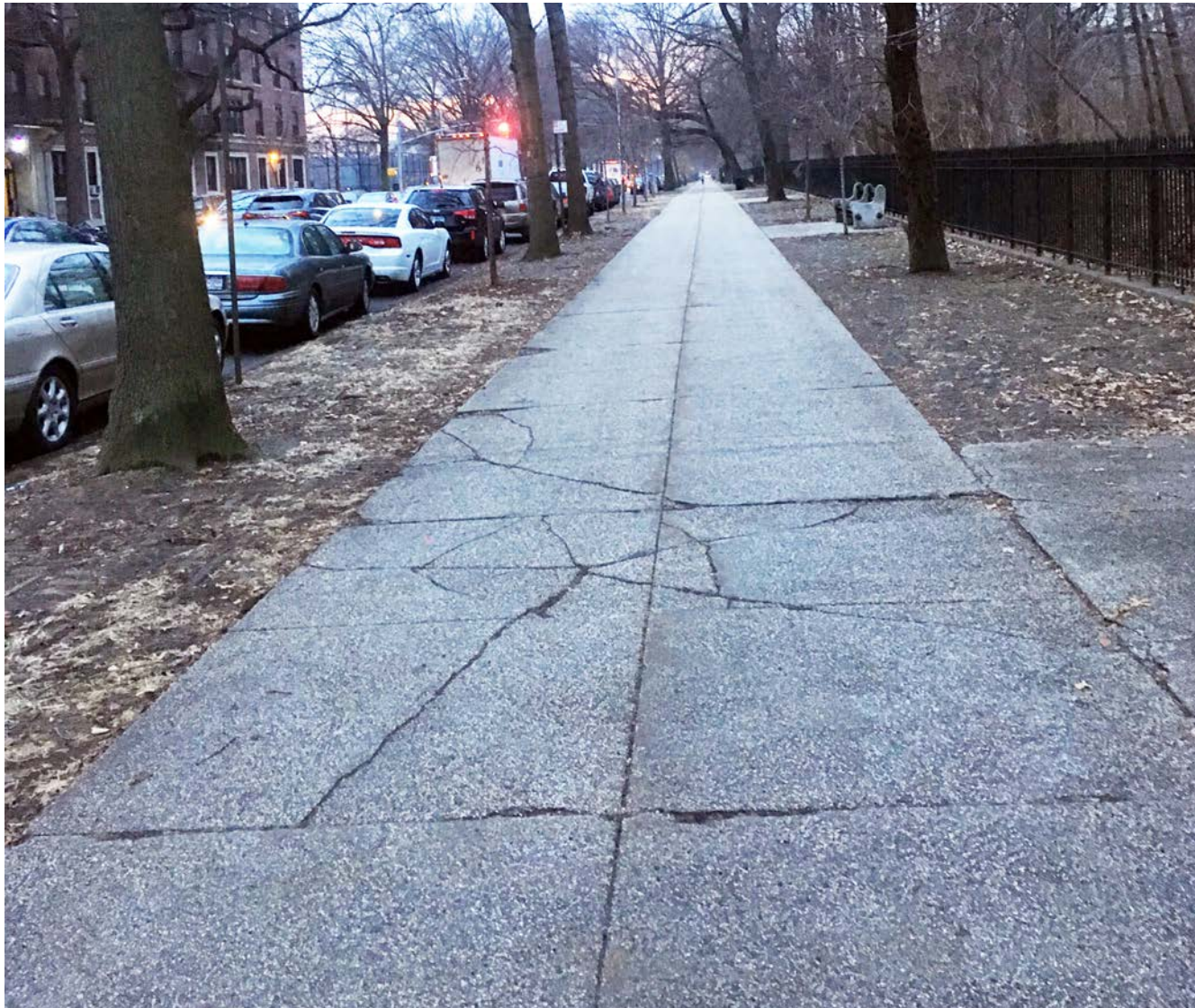
1 - Broken and uneven pavement
