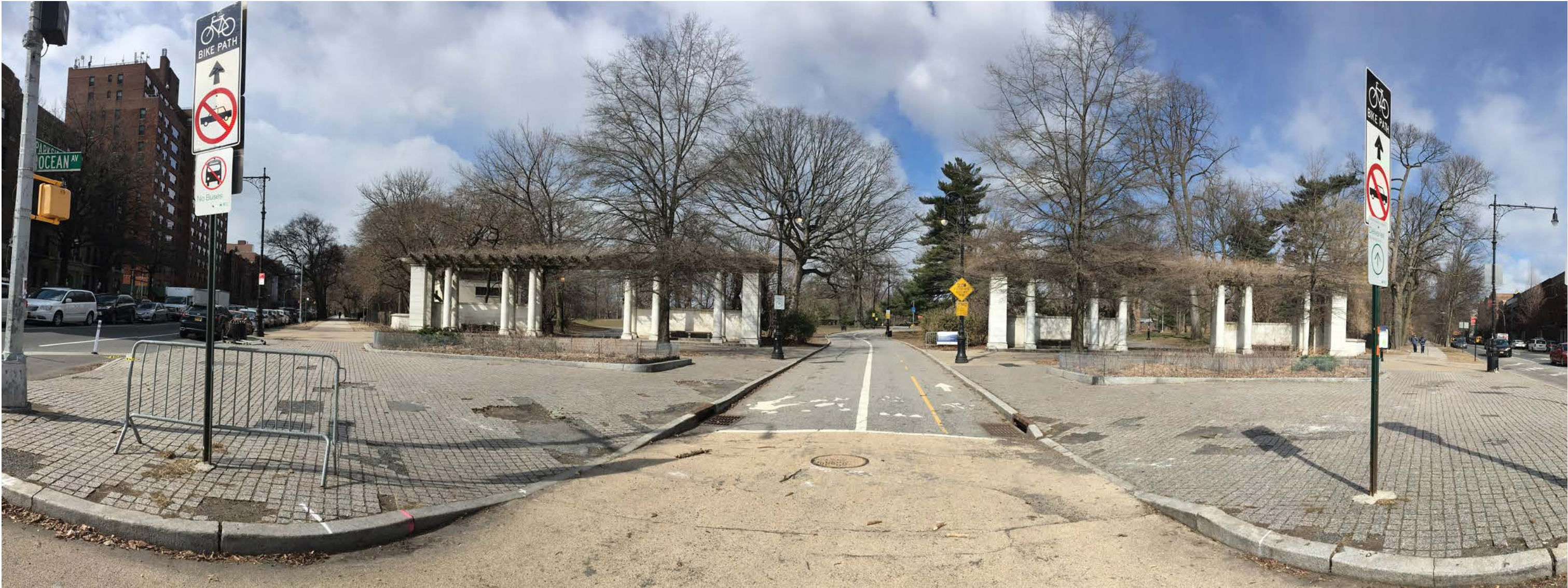
1 - Deteriorated Pavements, No Bike Lane, No Longer Used for Vehicular access
