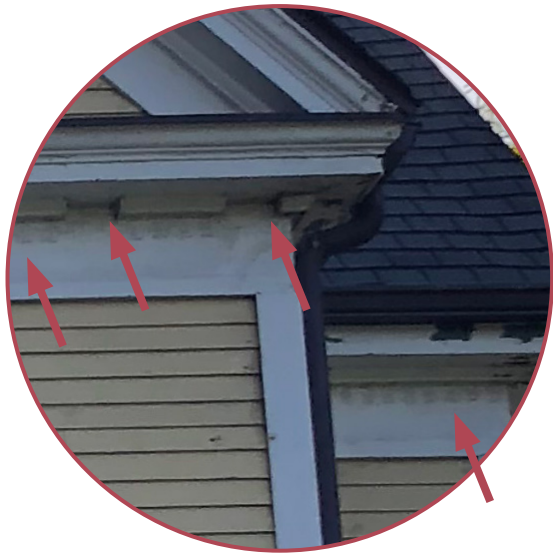
EXISTING CONDITION WITH MISSING BRACKETS AND DENTILS
