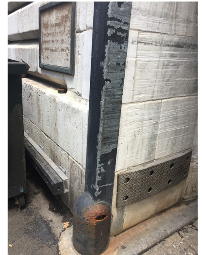
▲ 3 Damaged opening at primary Loading Dock entry
