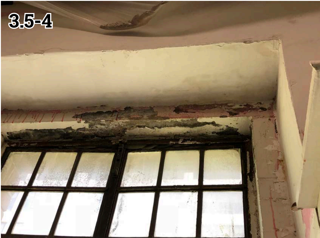
3.5-3 Interior Water Damage • Interior Damage Caused by Leaking Roof Above
