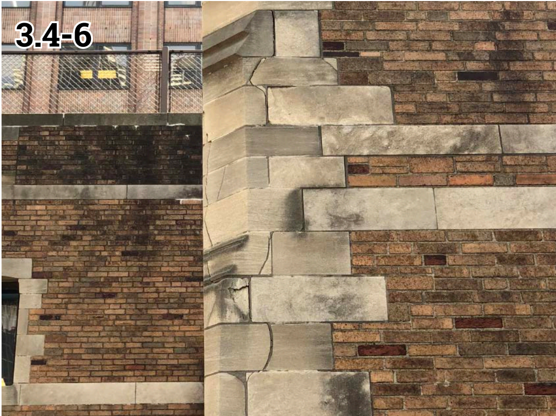
3.4-5 Parapet • Cracked Brick
