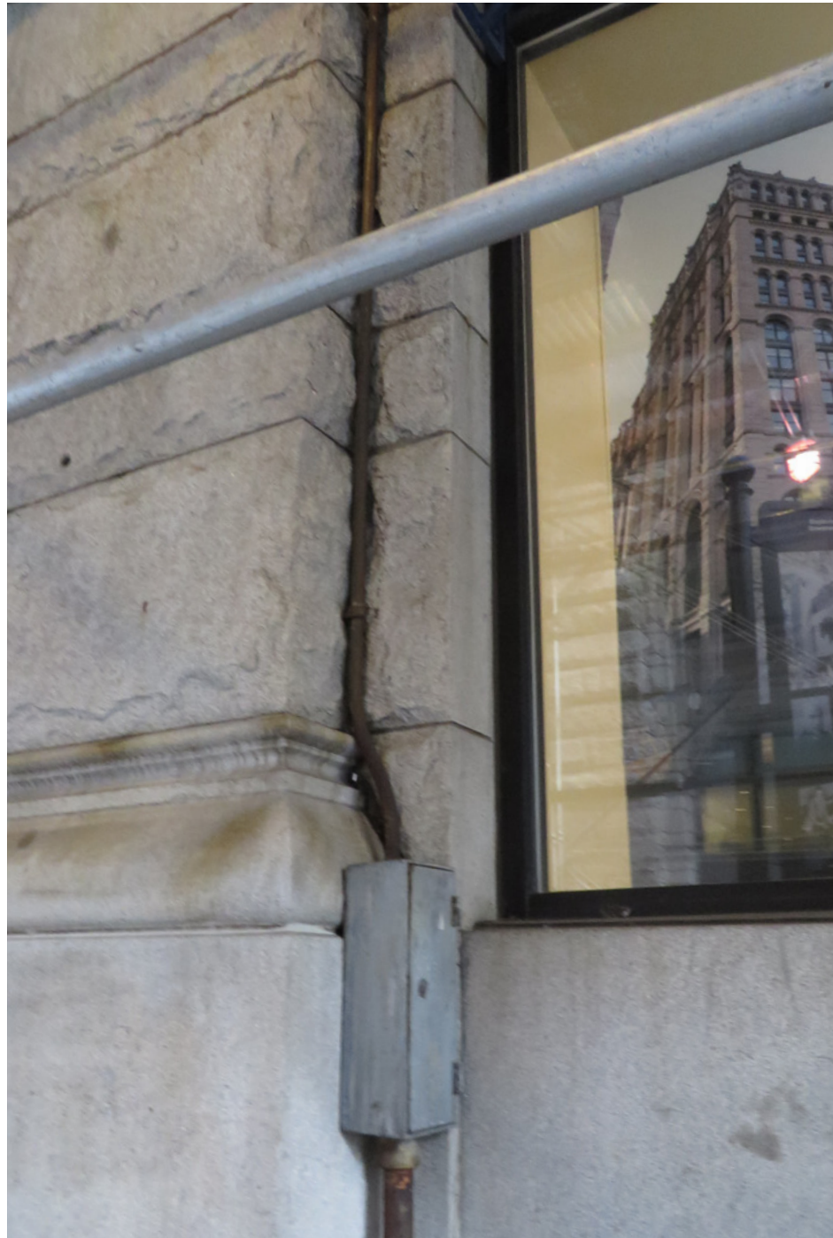
SURFACE MOUNTED CONDUIT TO EXTERIOR
