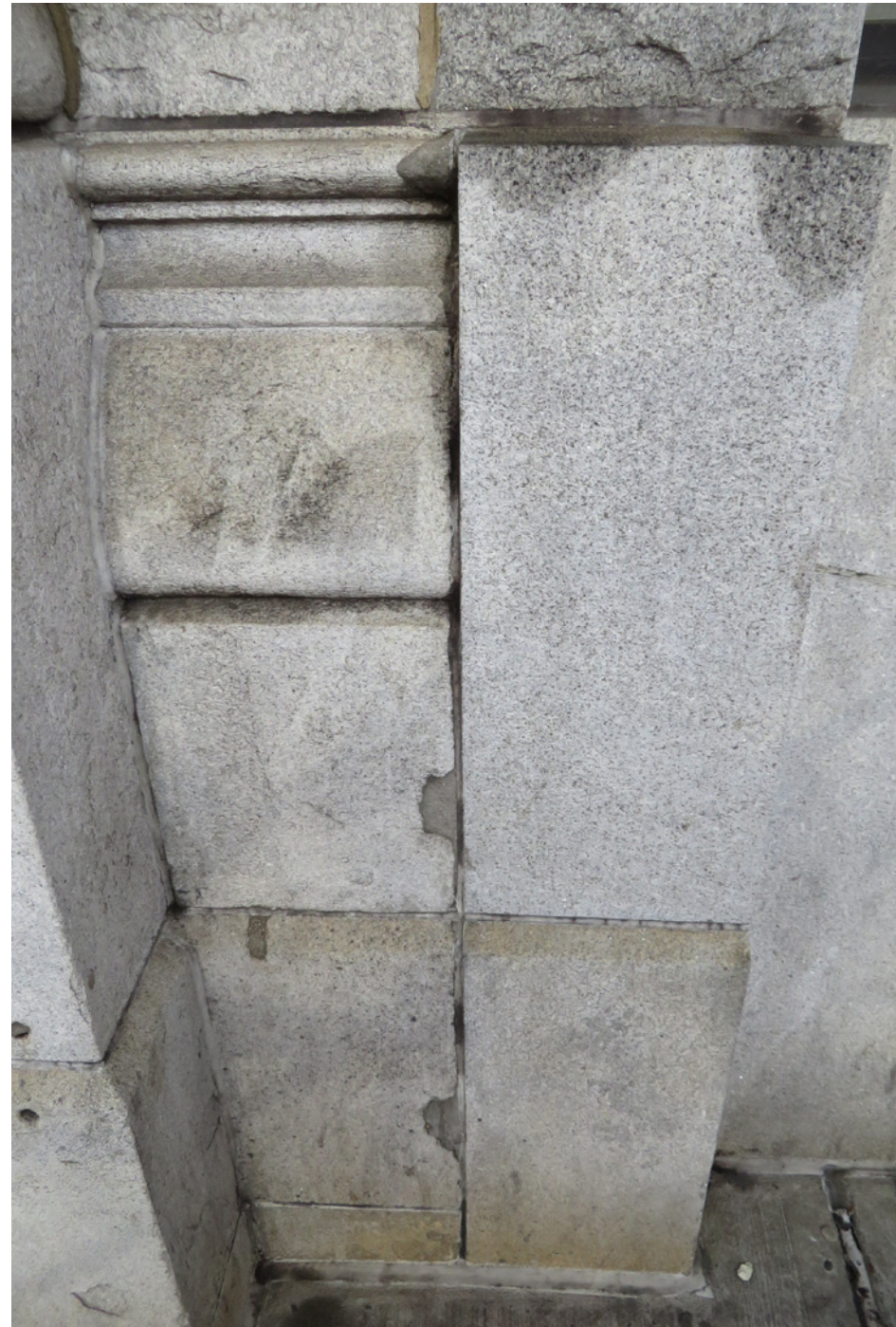
MODIFIED BASE AND SPALLING OF ORIGINAL GRANITE
