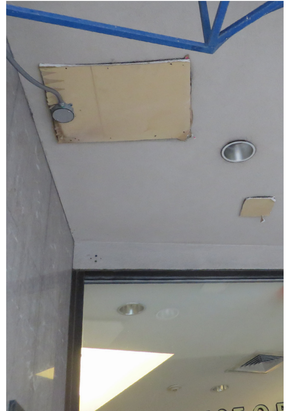
EXPOSED CONDUIT (AND PATCHED SOFFIT LINING)
