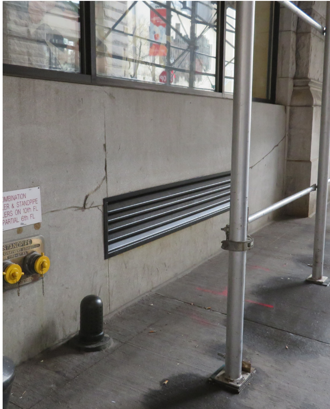
CRACKS IN GRANITE BASE (AROUND INFILL LOUVERS)
