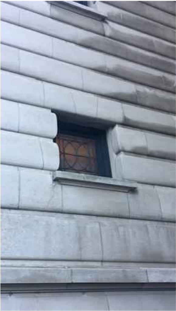
WINDOW REMAINING IN OWNERS APARTMENT
