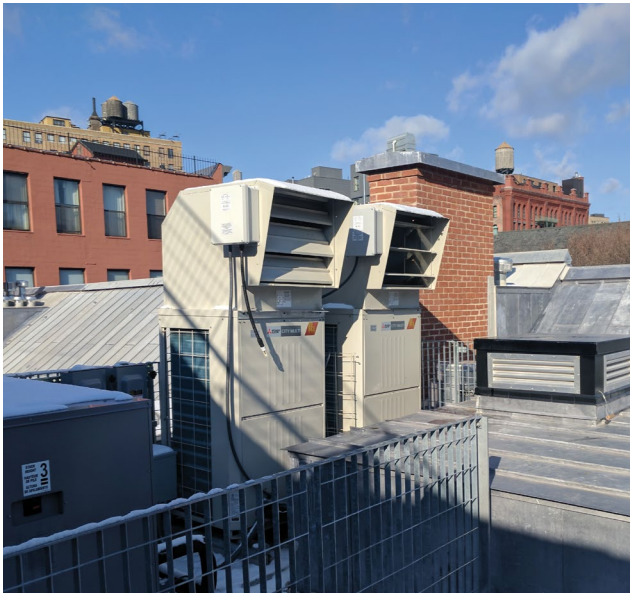
Rooftop HVAC installations, including vents and condensing units, can be minimally visible if it is not possible to make them non-visible from public thoroughfares.
