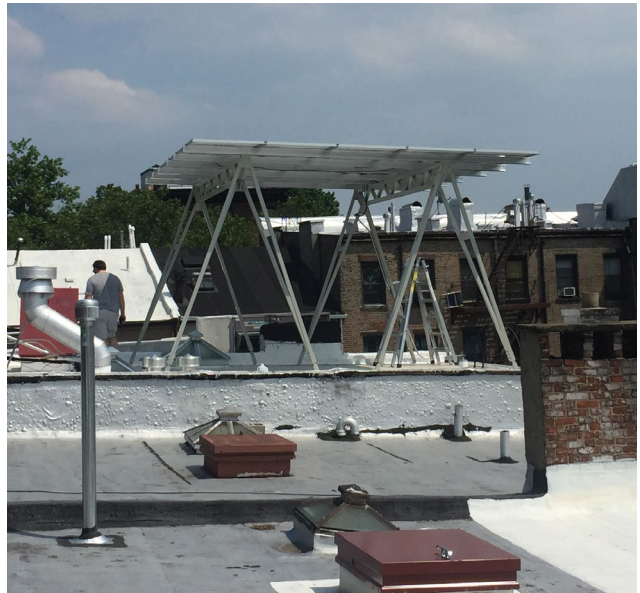
Rooftop installations can include other mechanical equipment like solar panels, as seen here.
