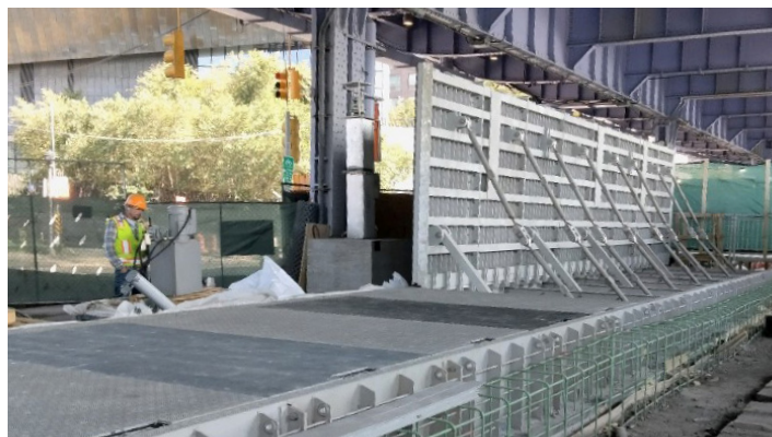
Flip up gates in partially-deployed position, Sept. 2024
