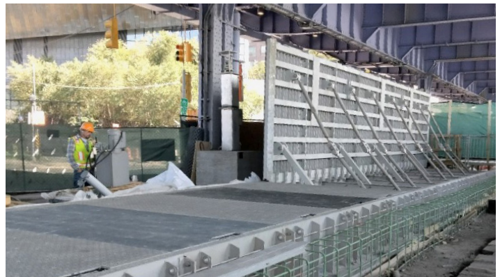
Flip up gates in partially-deployed position, Sept. 2024
