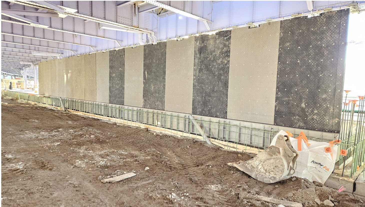
Flip up gate segments installed under FDR Drive near Robert F. Wagner Sr. Place – March 2026
