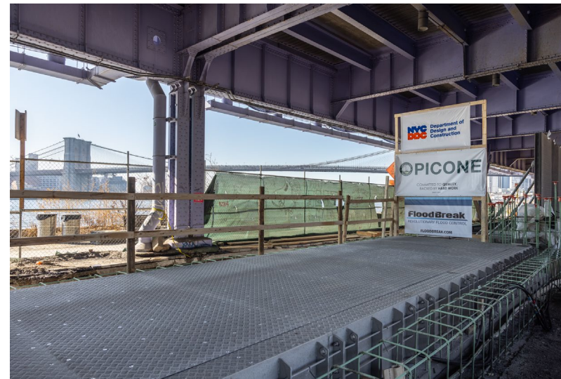
Flip up gate in closed position – March 2025
