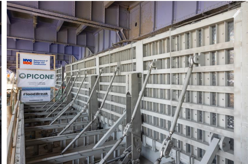
Flip up gate in open position – March 2025
