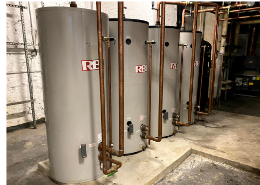
Split system indoor storage tanks
