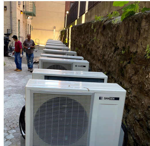
Split system outdoor heat pumps
