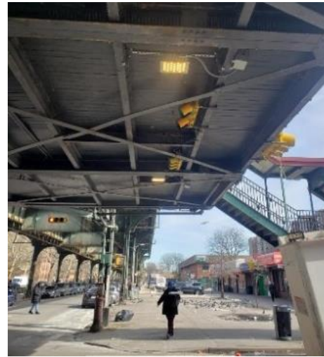
Underdeck lighting at Livonia Ave and Rockaway Ave
