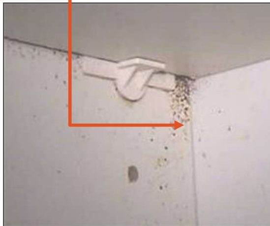
Cockroach dropping ("frass") under cabinets
