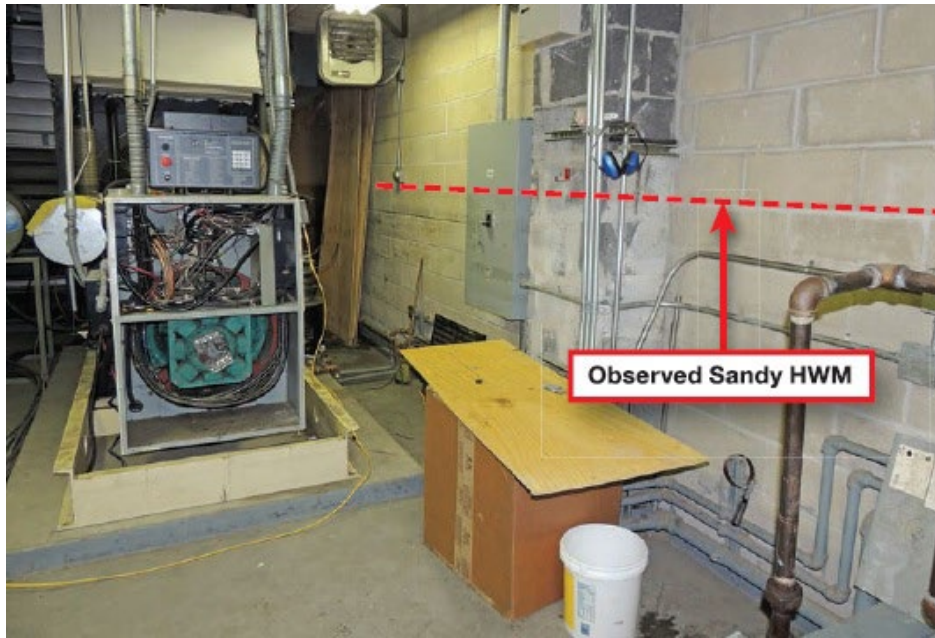
High Water Mark (red dashed line) along first floor electrical room wall.
