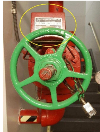
Tamper switch on a sprinkler valve
