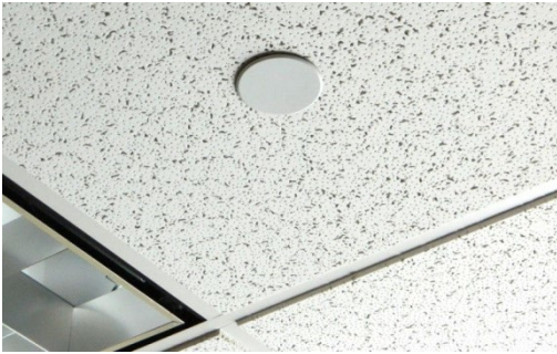
Concealed fire sprinkler heads with cover plates
