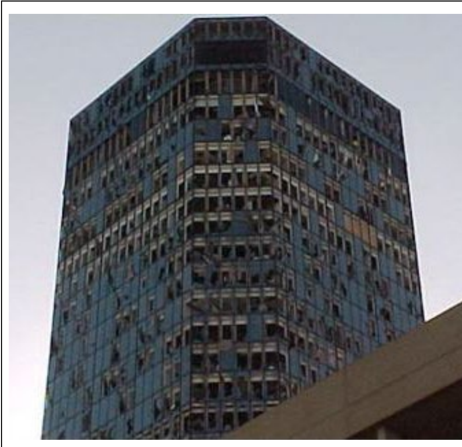
Windows and outer walls of the Bank One Building in downtown Fort Worth, Texas were damaged by the 2000 Fort Worth tornado.
