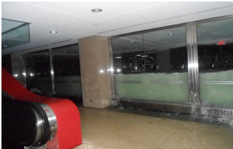
Hurricane Sandy storm surge filling the concourse retail level of a Manhattan commercial high-rise building
