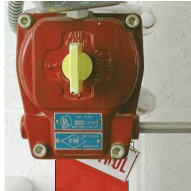
The picture shows the control valve is in the open position.
