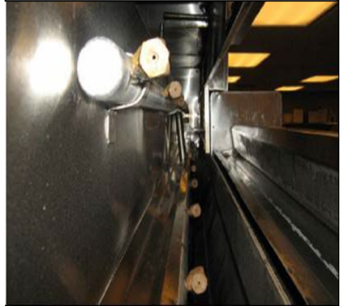
Nozzle installed in a water wash system hood
