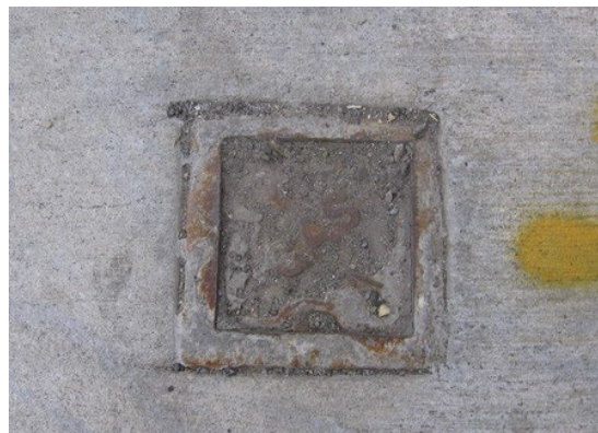
Gas shut-off valve in sidewalk
