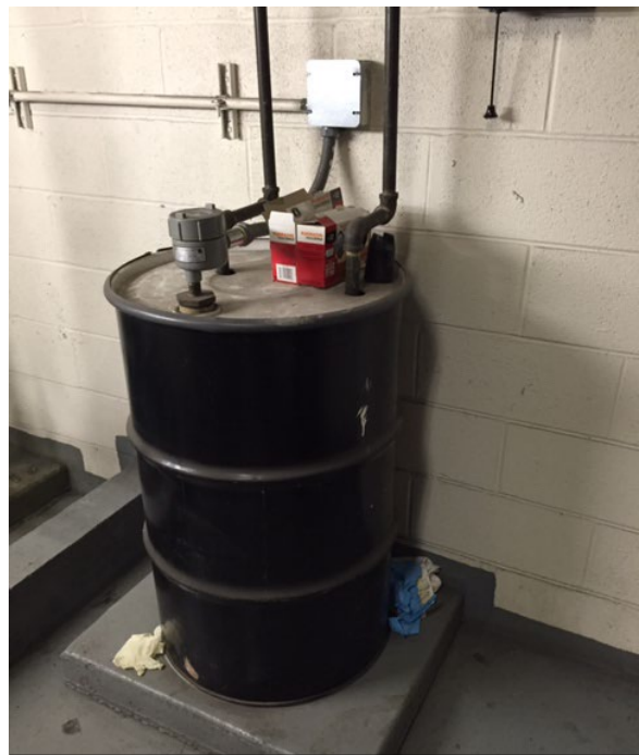
LEAK COLLECTOR WITH OIL LEVEL GAUGE
