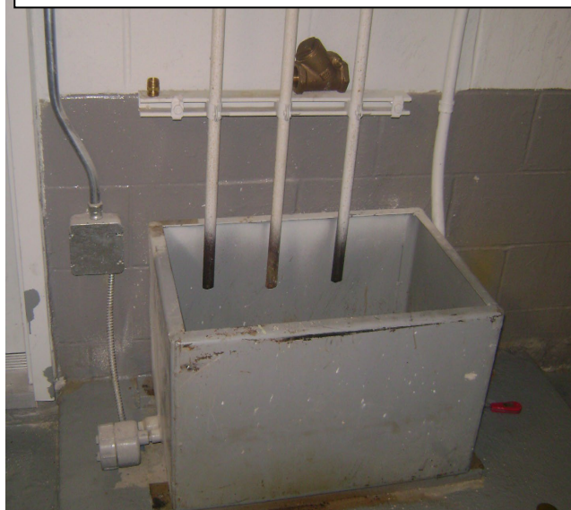
“Overflow Catch Basin” or tank with attached leak detection alarm
