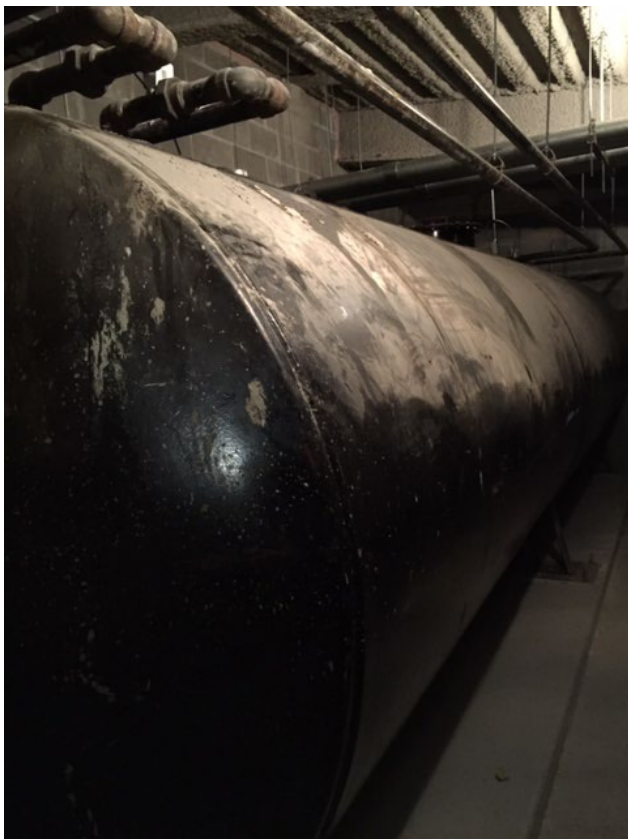
MAIN OIL STORAGE TANK ON THE LOWEST LEVEL
