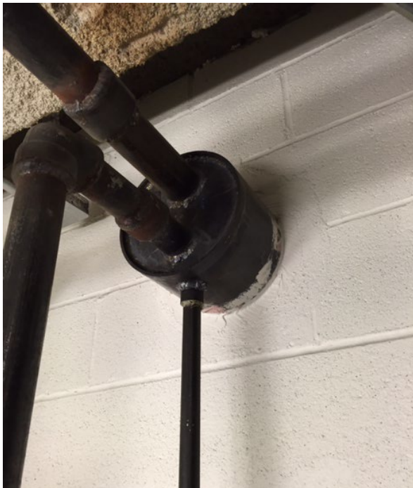
LEAK COLLECTOR INSIDE THE WALLS
