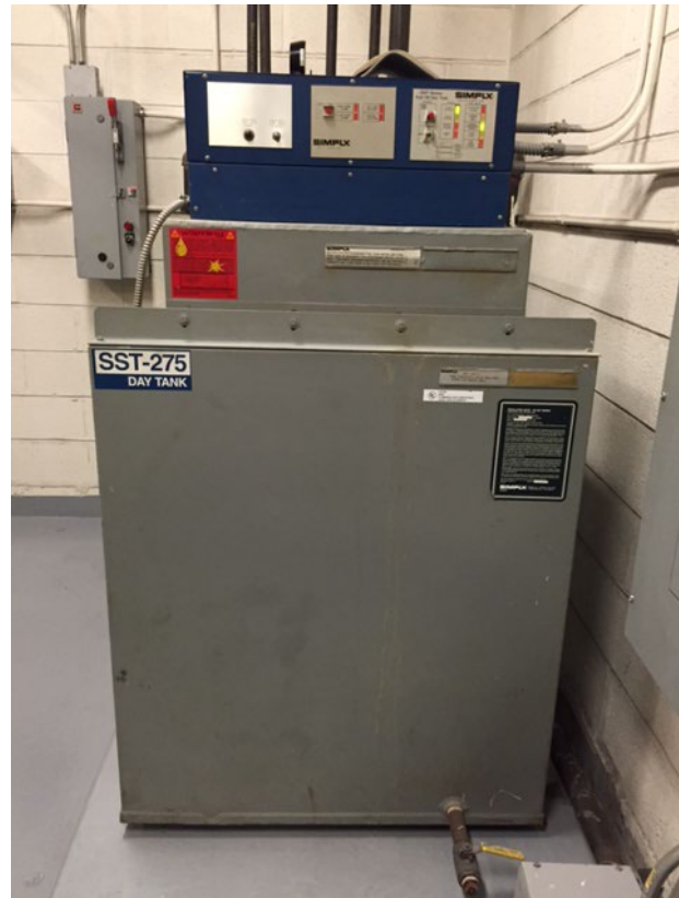
DAY TANK INSIDE A DIKE
