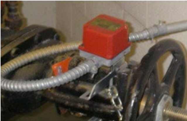
Tamper switch on a sprinkler valve
