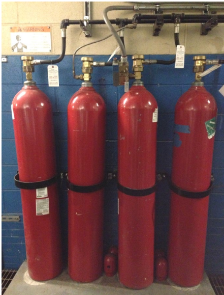
CO 2 fire suppression system cylinders
