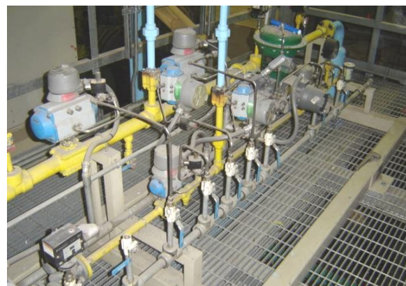
Duct Burner Gas Train
