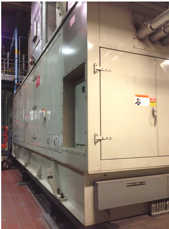
Gas Turbine-Generator Enclosure
