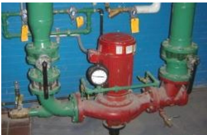
Typical Cooling Water Pumps
