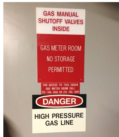
Example of Warning Sign outside the Gas Meter Room
