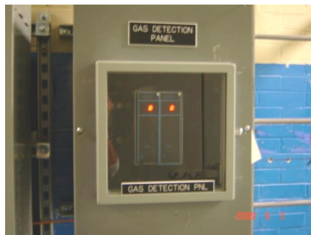
Gas Detection Panel
