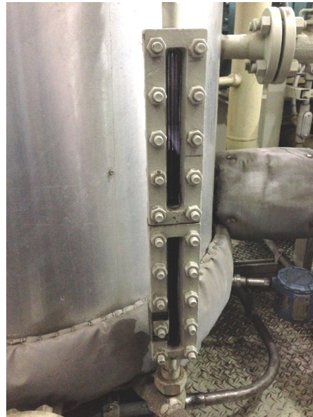
Monitoring Oil Level in Separator Tank
