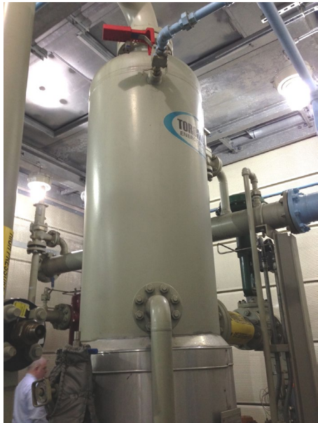
A Gas-Lube Oil Separator
