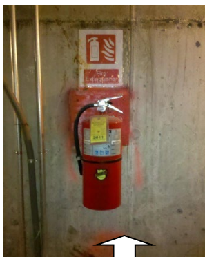
Fire extinguisher in a construction site
