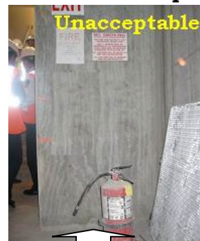
Improper floor placement of Fire Extinguisher.
