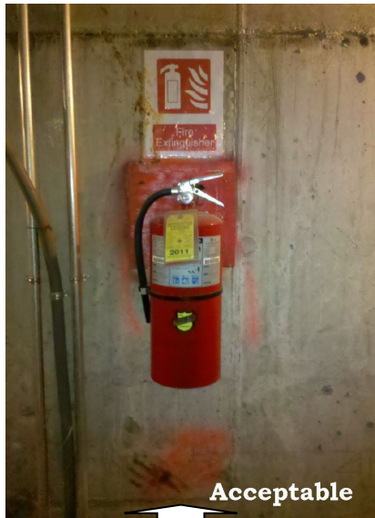
Acceptable Fire extinguisher in a construction site.
