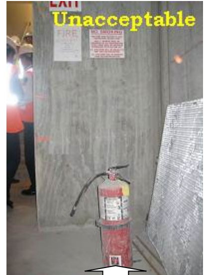
Unacceptable Improper floor placement of Fire Extinguisher.
