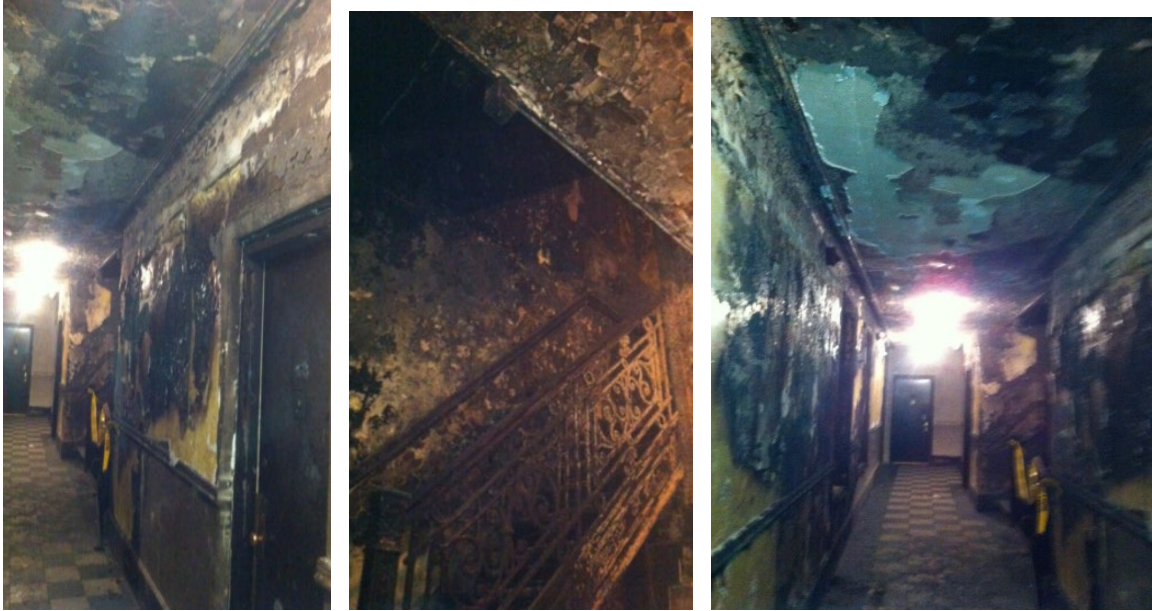
Pictures show the interior of the Bronx, NY shelter after the second mattress fire. There was severe smoke and fire damage in the hallways and stairwells.
