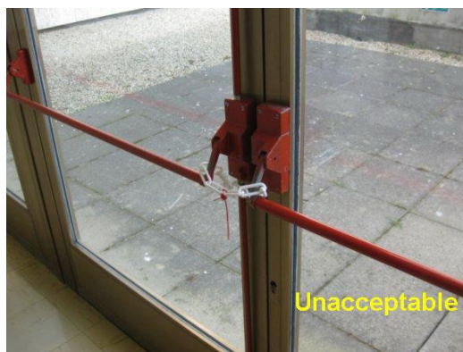
Picture shows a chained exit door, which is unacceptable.
