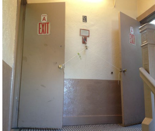
Fire doors illegally suspended open
