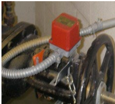
Tamper switch on a sprinkler valve
