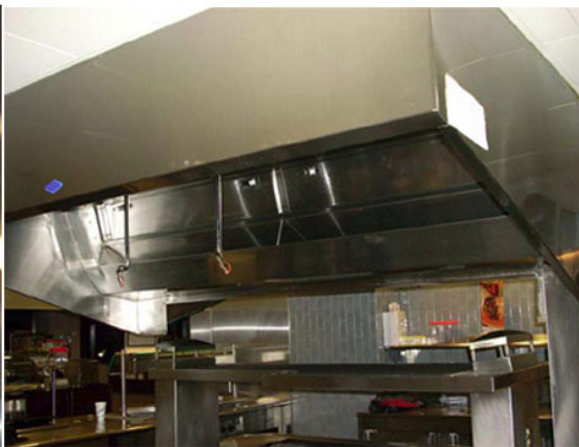
TYPE I HOOD WASH HAS PLENUM DOORS
