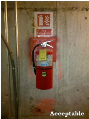
Fire extinguisher in a construction site.
