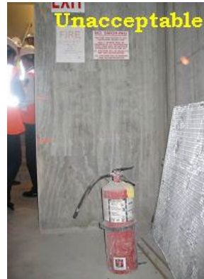
Improper floor placement of Fire Extinguisher.
