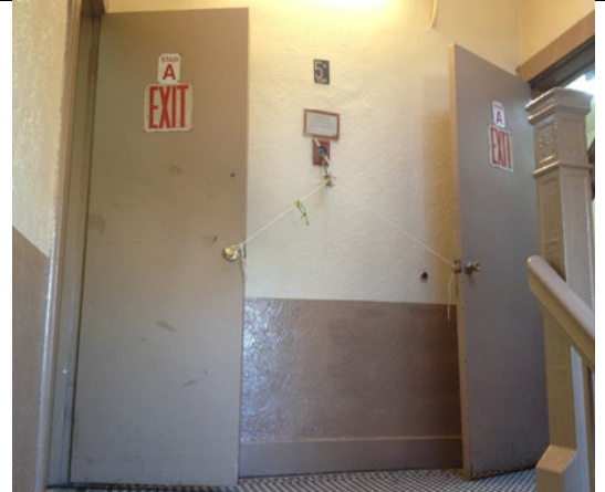
Fire doors tied open ( illegal )
