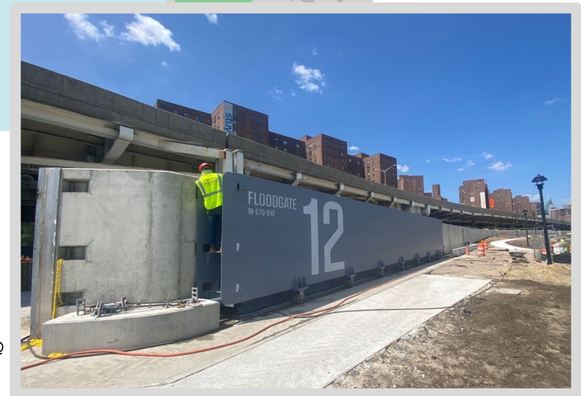
Flood Gate 12 installed at Stuyvesant Cove Park @ E. 20 th Street entrance
