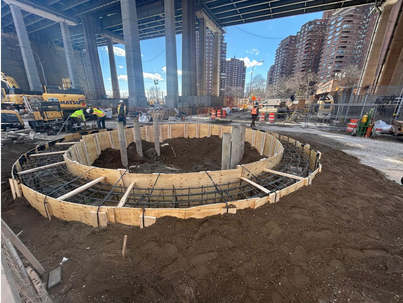
Cap beam installation for deep drop manhole on Delancey St. North – April 2026
