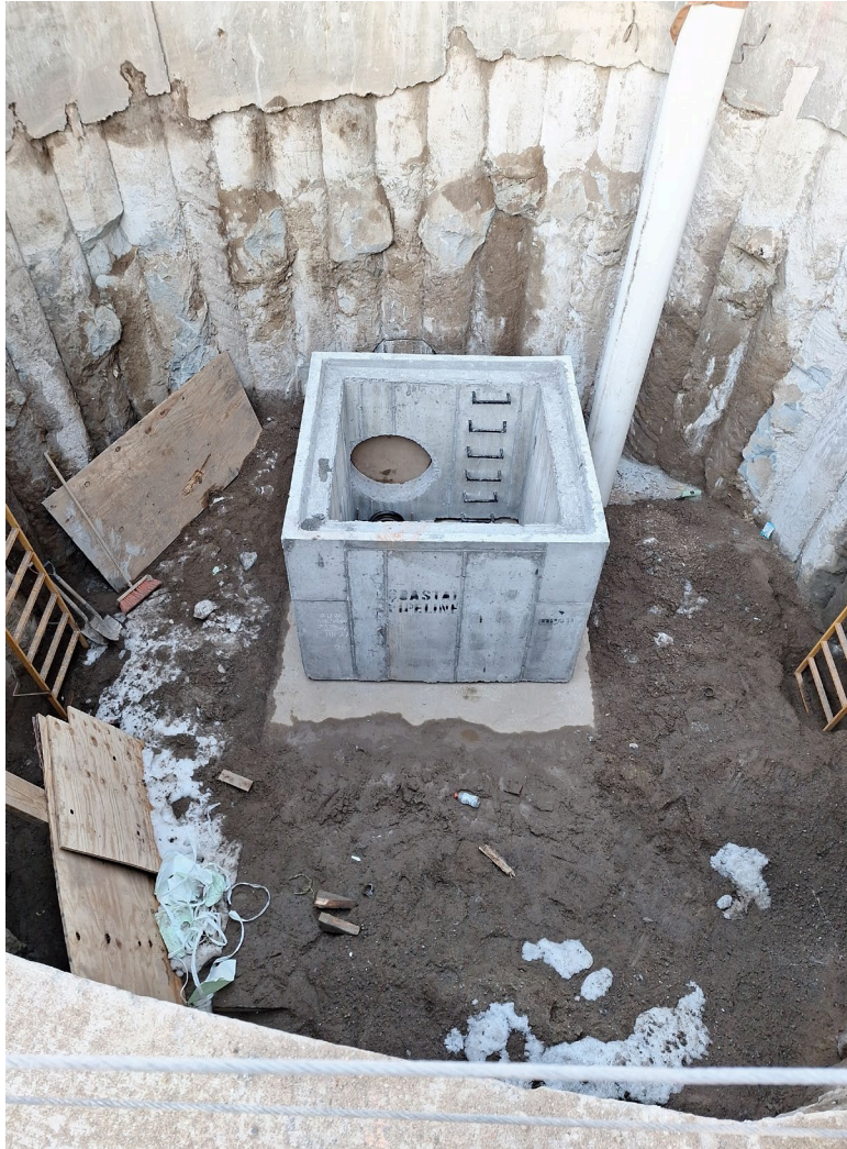
Deep drop manhole in Delancey Street South and Baruch Drive – March 2026
