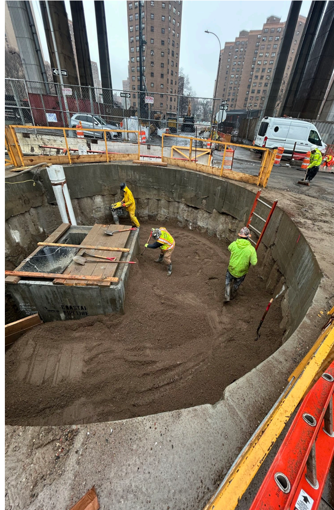
Backfilling of deep drop manhole in Delancey Street South and Baruch Drive – March 2026
