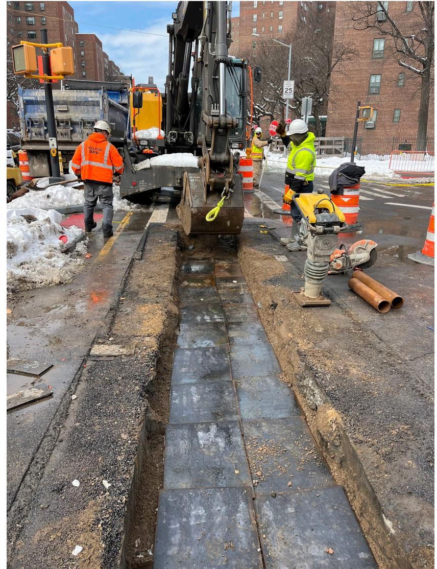
Installation of steel plates for utility conduits on E. 20 th Street – March 2026
