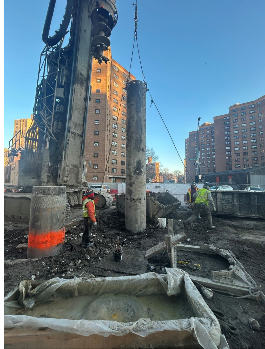
Secant pile installation for Deep Drop Manhole at Delancey Street N and Baruch Dr. – February 2026
