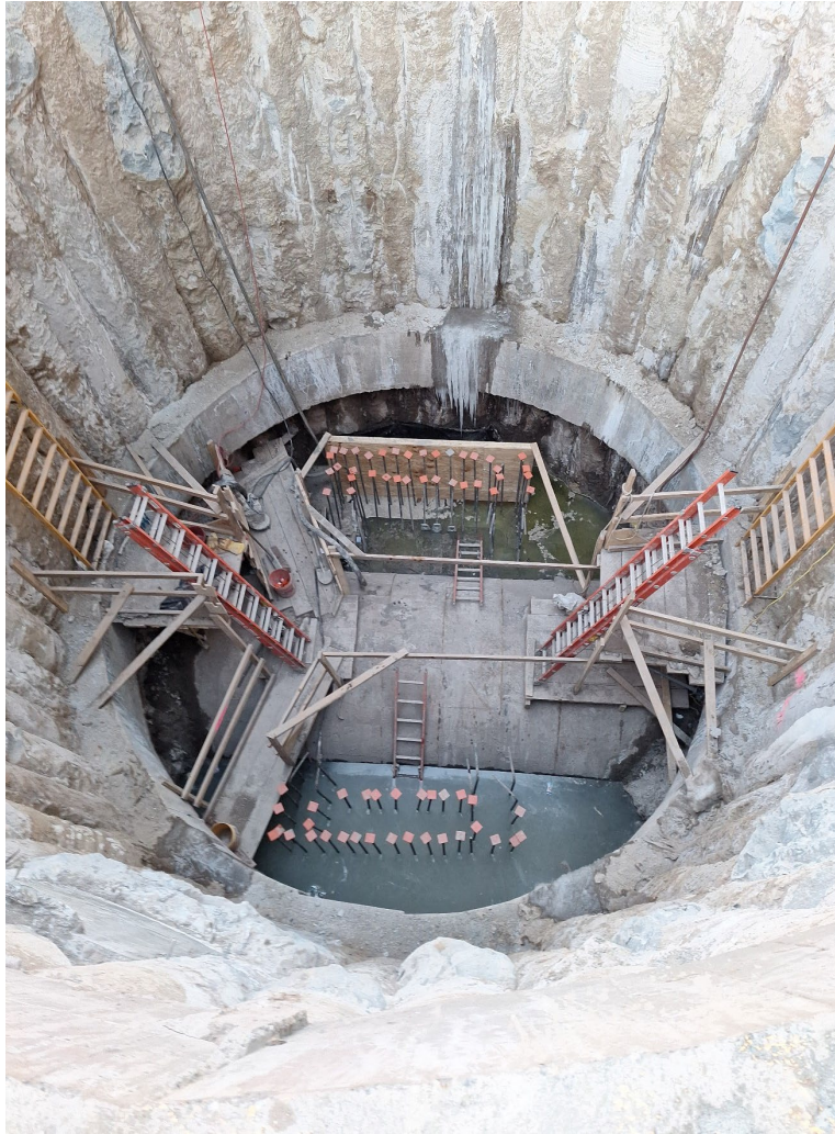
Formwork for Deep Drop Manhole installation at Delancey St. S and Baruch Dr. – February 2026
