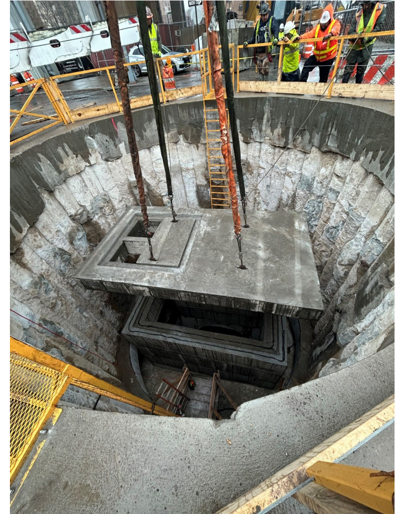
Deep Drop Manhole roof slab installation at Delancey St. S and Baruch Dr. – February 2026
