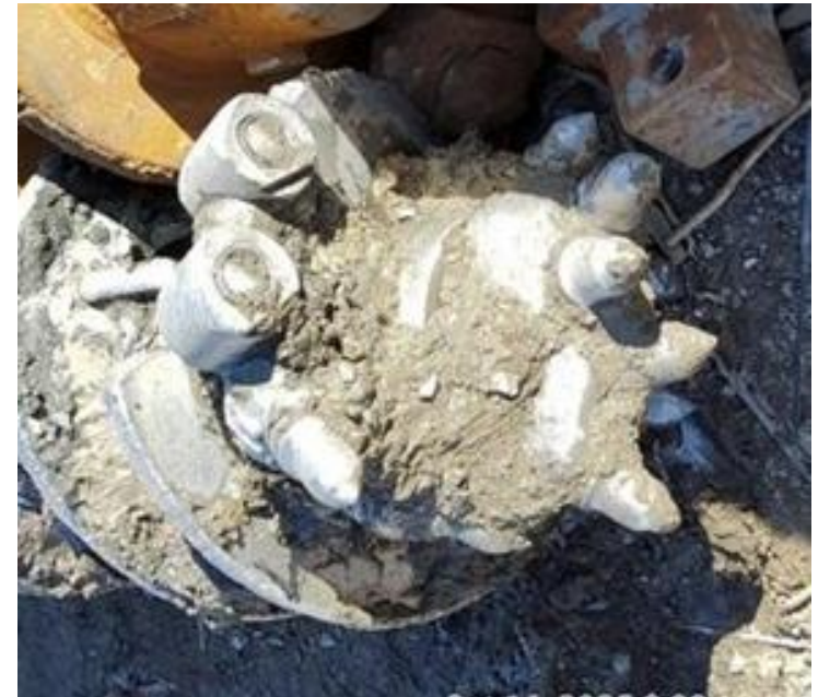
Drill bit teeth damaged by obstructions
