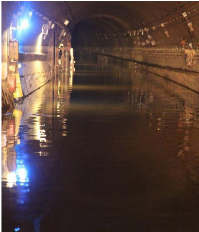
FLOODED SUBWAY TUNNEL FROM HURRICANE SANDY
