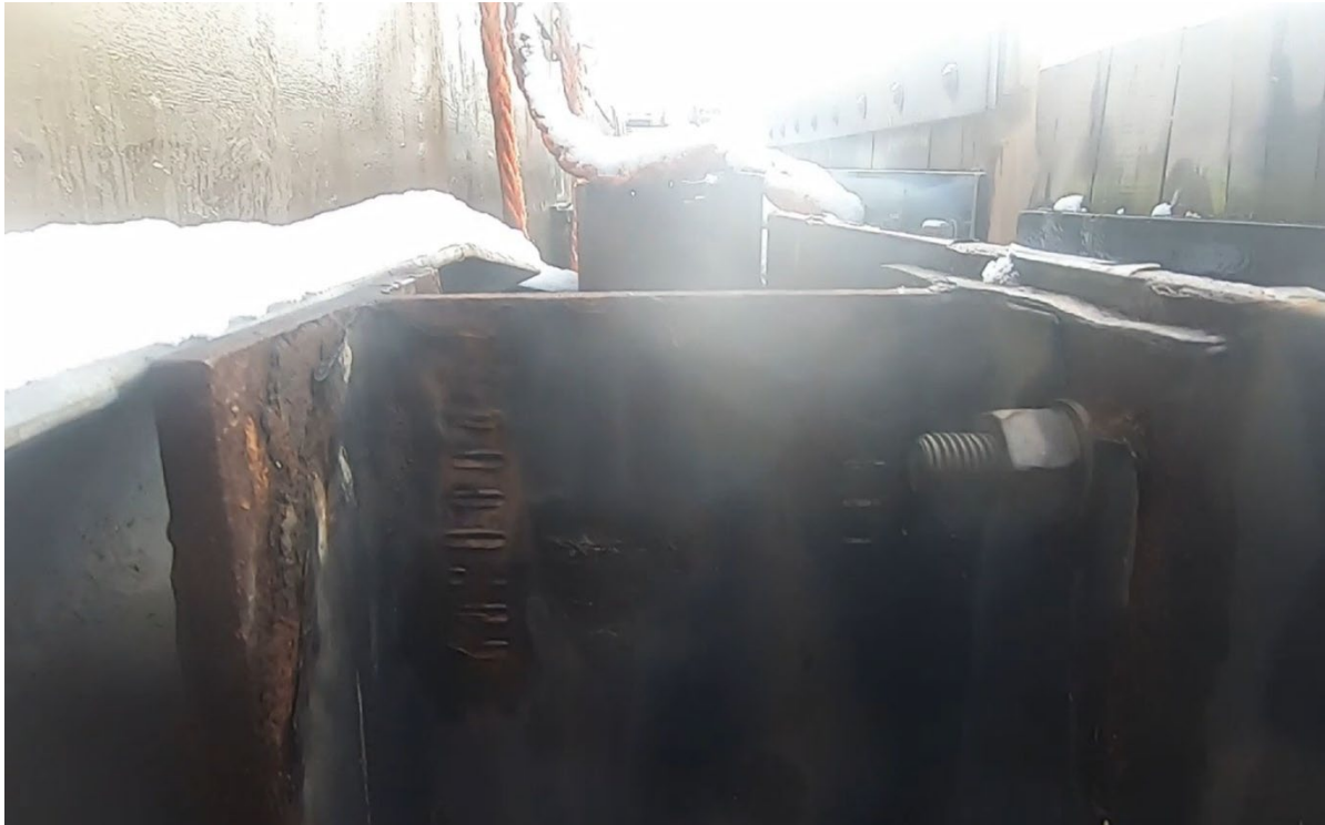
Photo 5: Fender pile with heavy coating loss & moderate corrosion at top of pile. Corrosion of flange edges continues further down.
