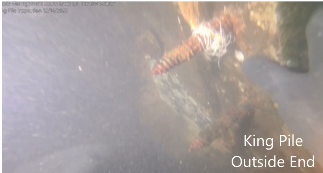
Photo 23: Exposed lag bolts at missing timber support / fender.
