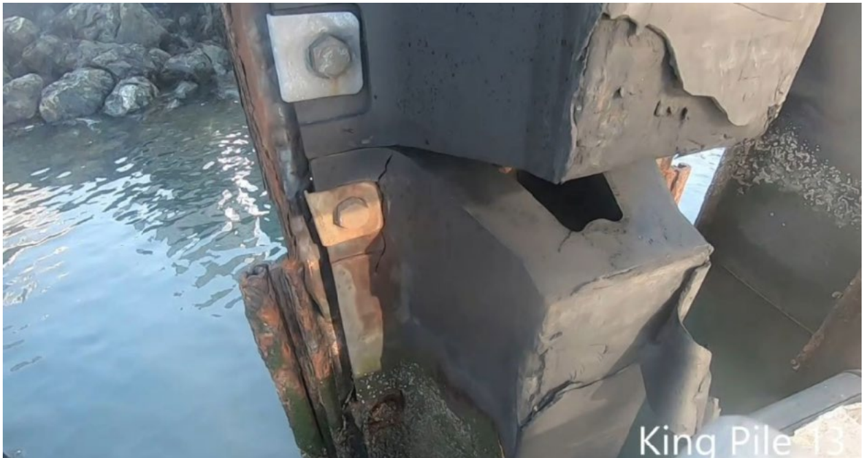
Photo 22: Typical fender damage (King Pile 13).
