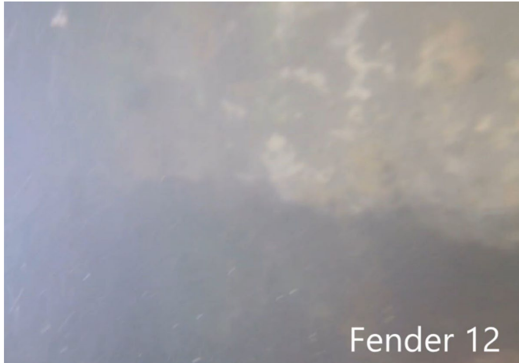
Photo 15: Typical below water concrete repair (turbidity prevented clear imagery).
