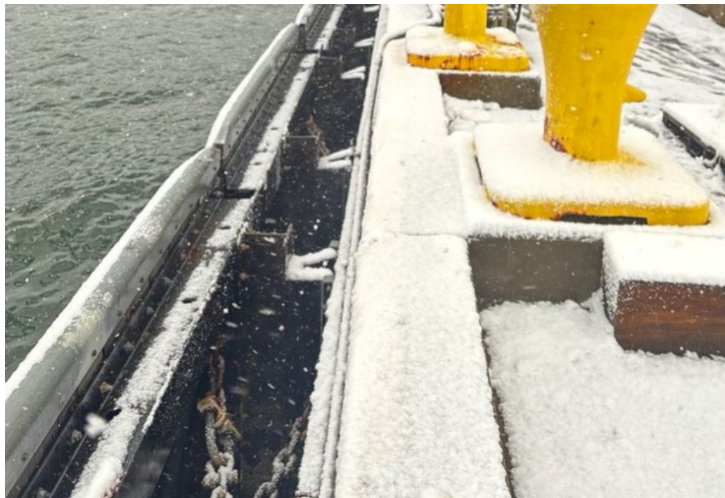
Photo 16: Typical Condition of concrete curb behind Fender #s 15 thru 20
