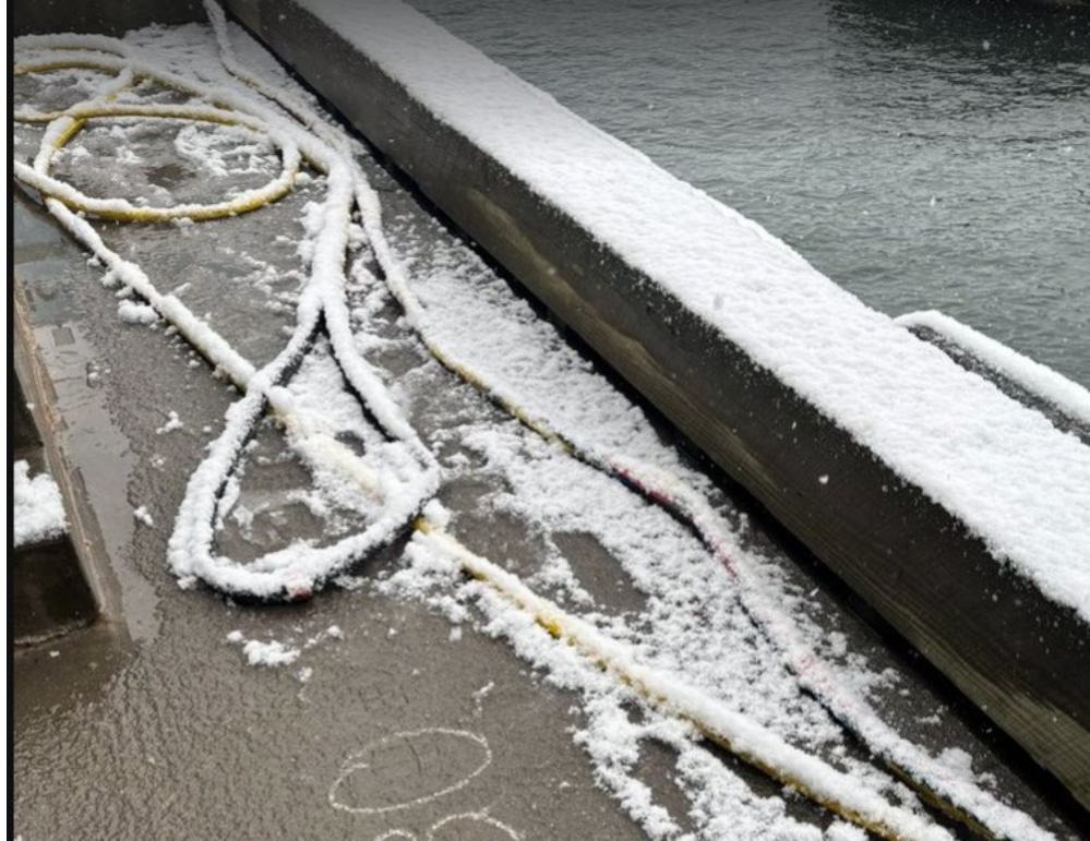
Photo 17: Typical condition of timber curb behind Fenders #1 through #15.
