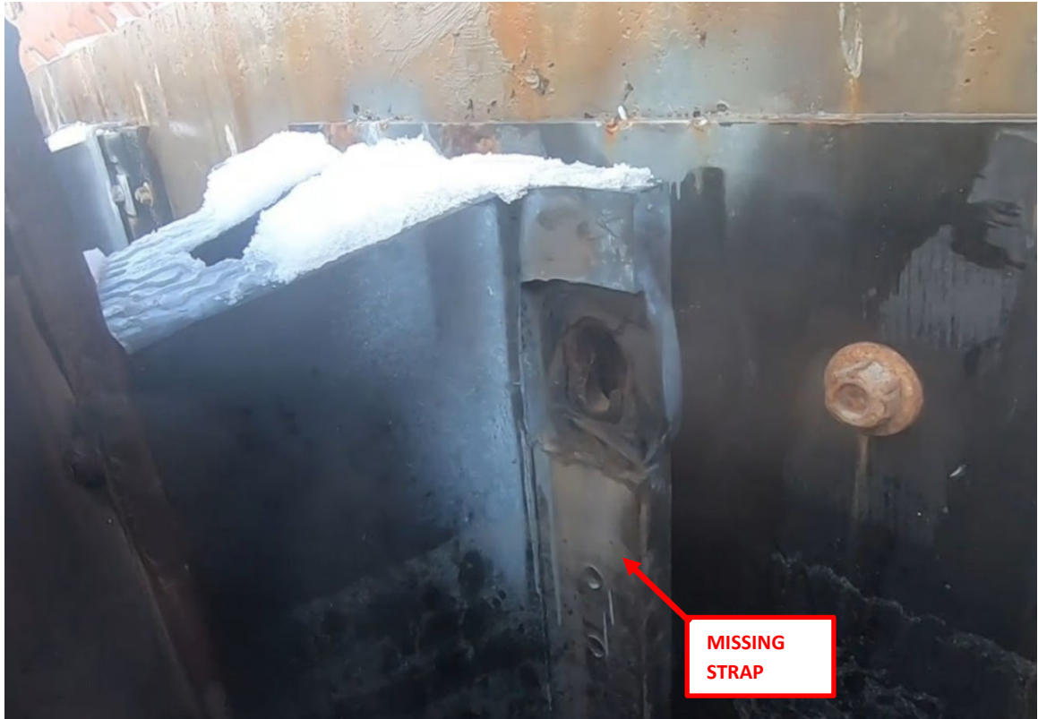
Photo 4: Strap repair failure at Fender #19.
