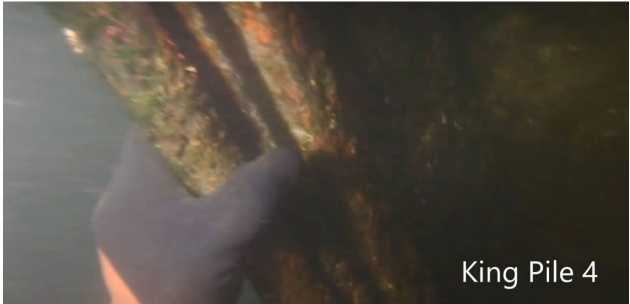
Photo 19: Typical condition of Sheet Pile (divers' hand is on interlock).
