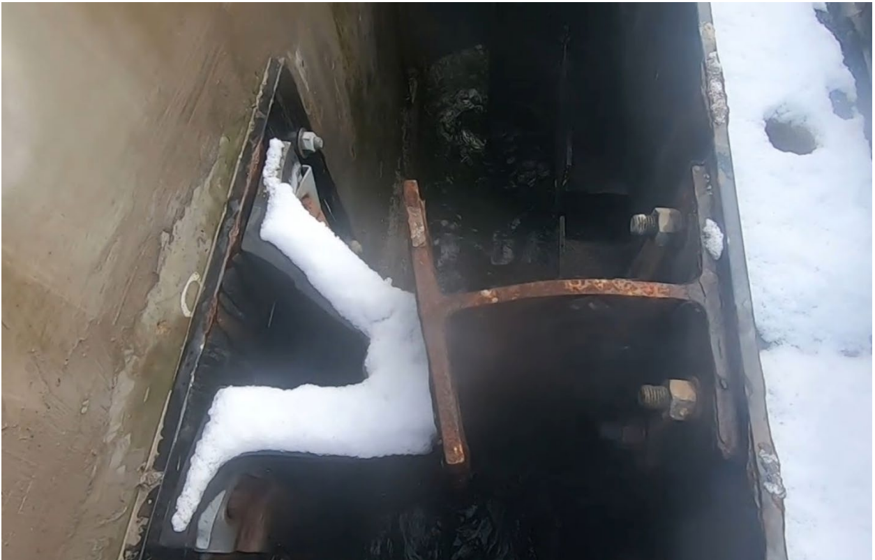
Photo 7: Deflection of Fender 9 South Pile.
