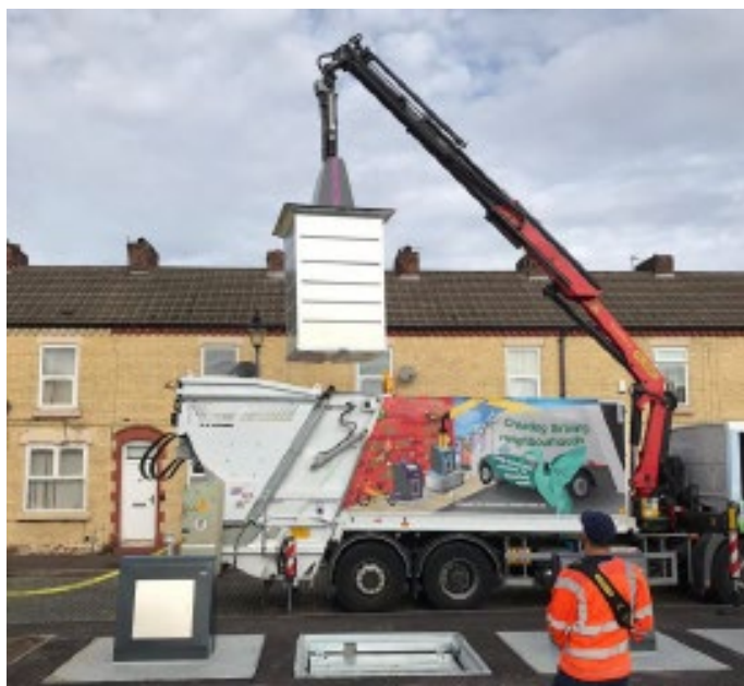
Photo #15. Example of Hoisted Waste Collection from an Underground Storage System
