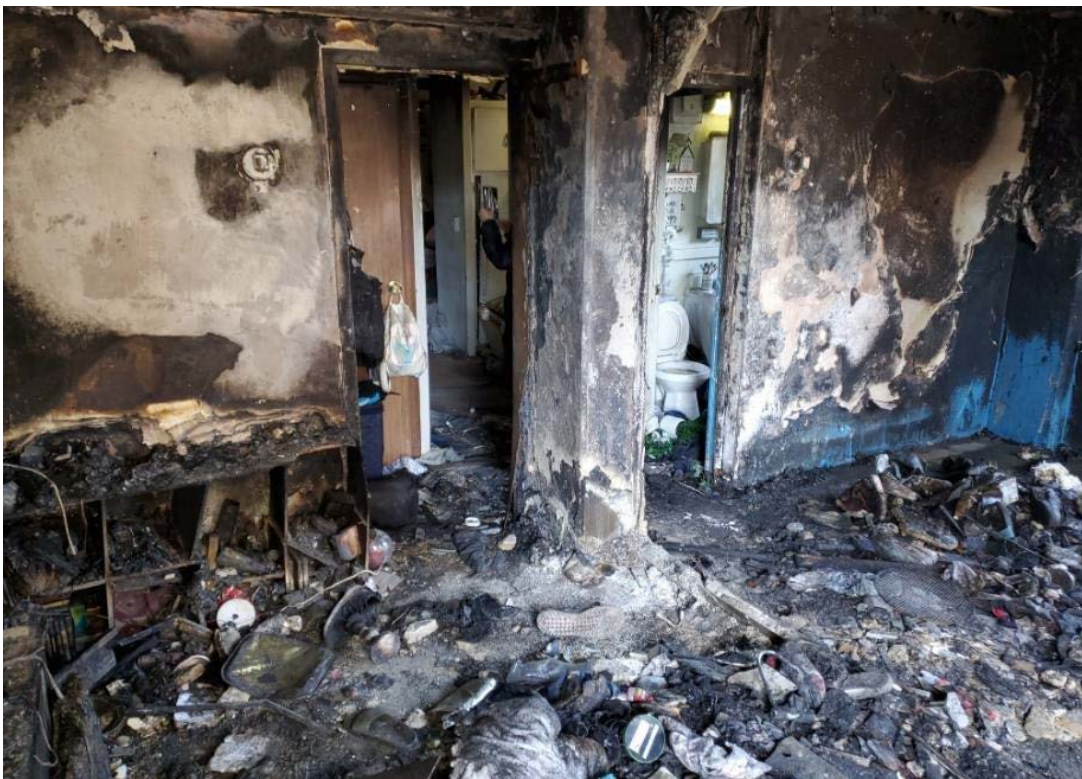
Charred remnants of the non-load bearing wall in the subject apartment; building B10, Riis Houses. Photo courtesy of FDNY BFI.
