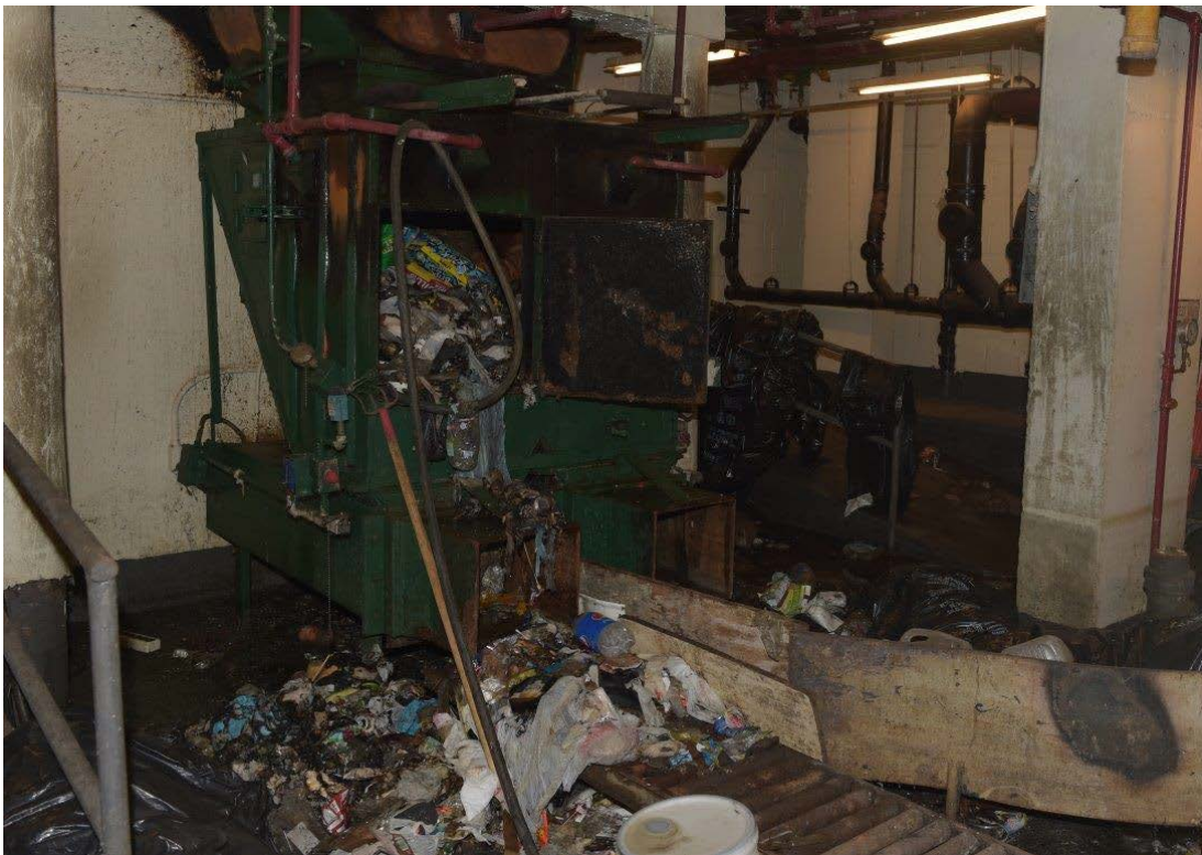
Compactor; building B1, Mitchel Houses. Photo courtesy of FDNY BFI.
