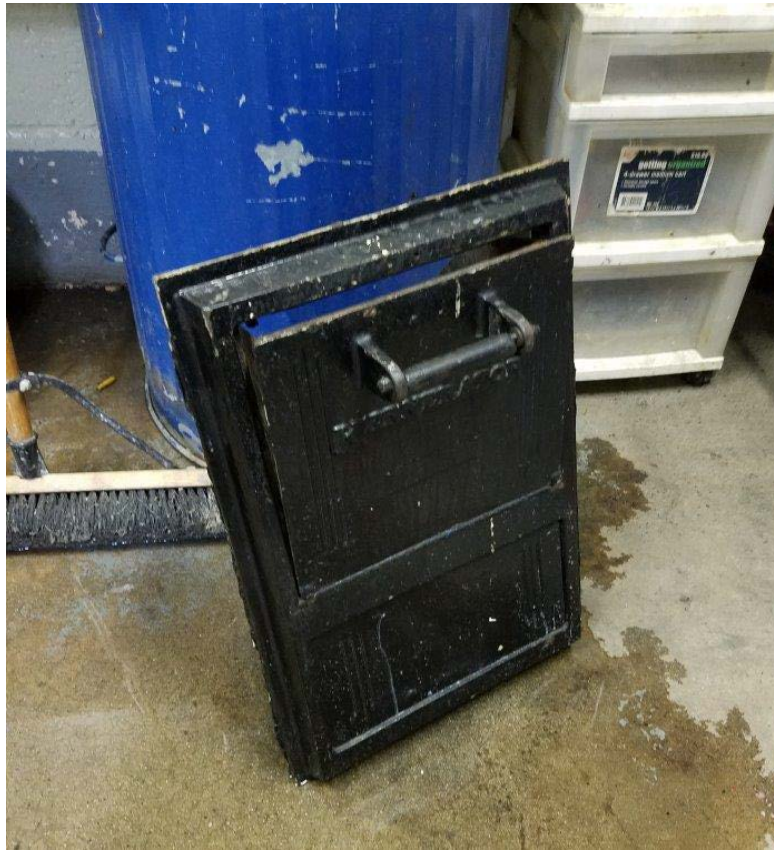
Hopper door detached from chute opening; building B2, Wise Towers. Photo courtesy of FDNY BFI.
