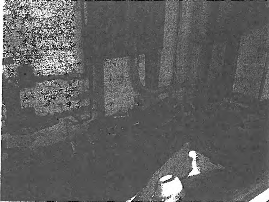
M13. Backflow Preventer
