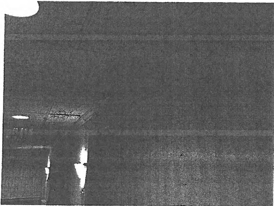
M18. Corridor Emergency Light
