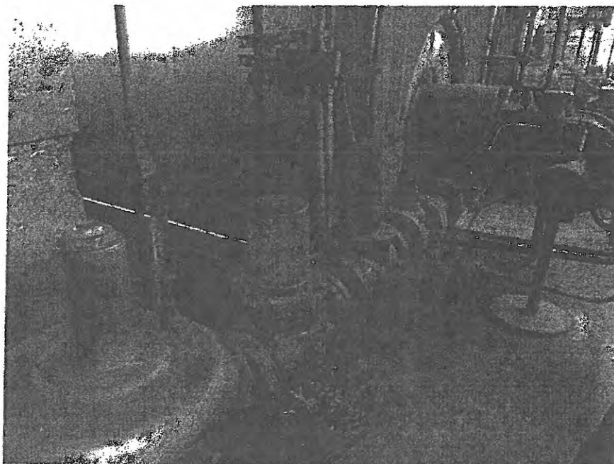
M3. Boiler Gas Train
