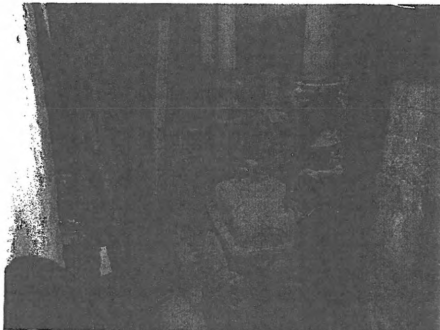
M5 Gas Service and Gas Meters
