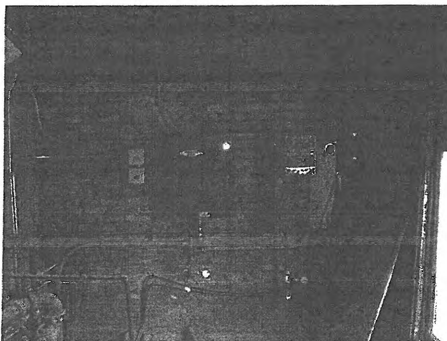
M26. Fire Pump Control Panel
