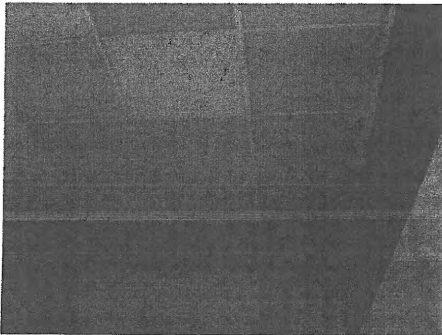
10. Close-up of rusty edge at entrance canopy
