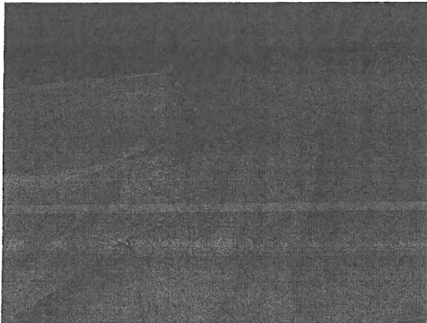
16. Bubbled roof surface at northwest corner of main roof
