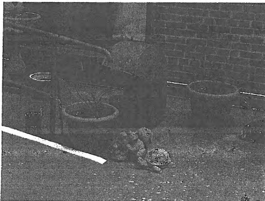
M10. Damaged Intake 2 Hood - 2nd Floor Roof
