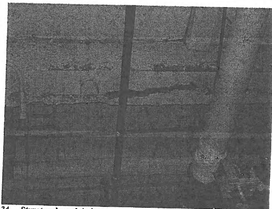
34. Structural crack in beam at ceiling above boilers
