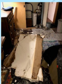
Pictured: Collapsed Roof
