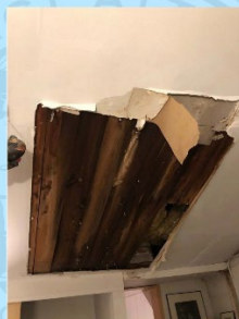
Pictured: Damaged Roof
