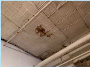
Pictured: Water Damage and Rust
