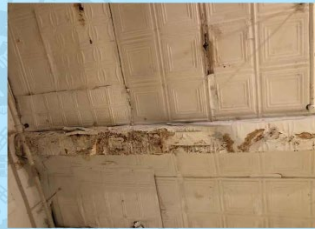
Pictured: Water Damage and Rust
