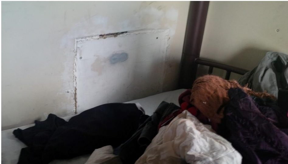
Figure 5: A cluster resident's bedroom that is not slept in. She told DOI that roaches crawl in through the crack in the wall.
