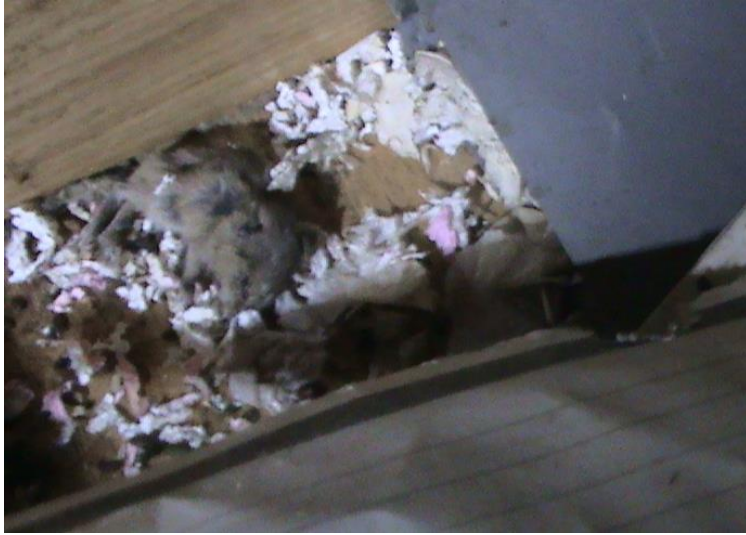
Figure 8: Mike's House (hotel): Dead mouse in a drawer of one of the units.
