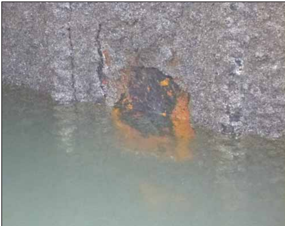
Photo 38-Deteriorated area on south side of steel sheet pile bulkhead
