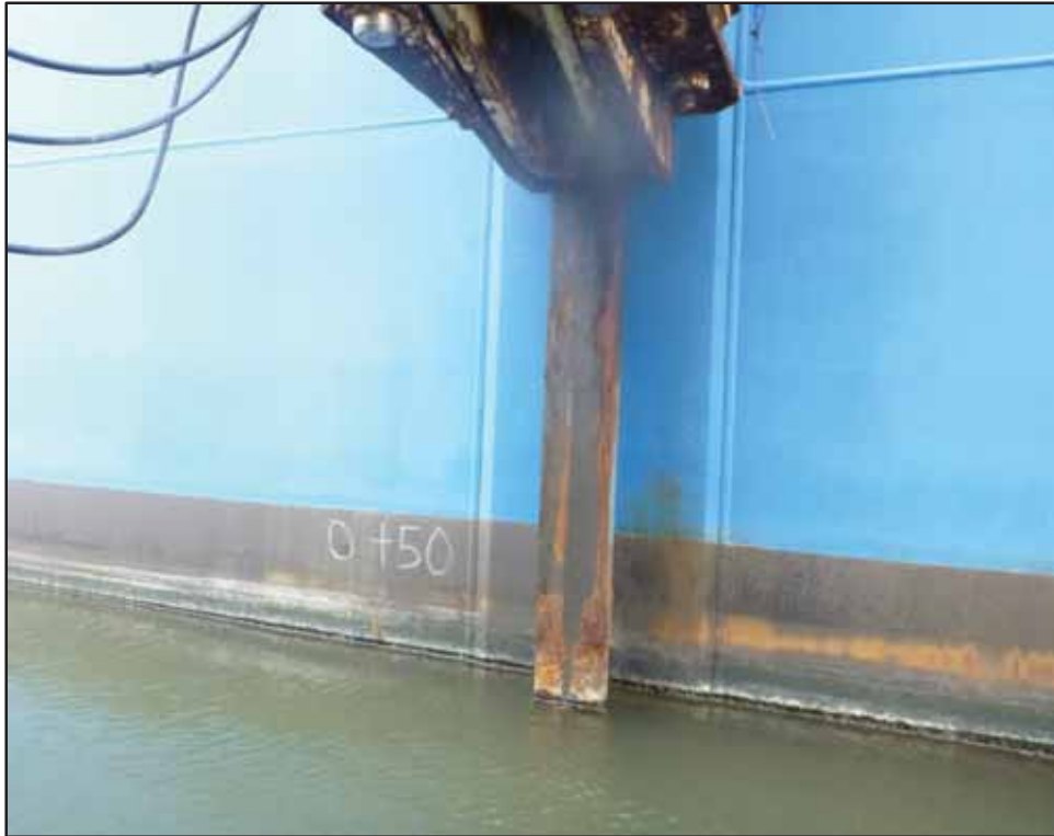
Photo 9-Corrosion of T-Beam in splash zone of single mooring connection at Station 3 + 22
