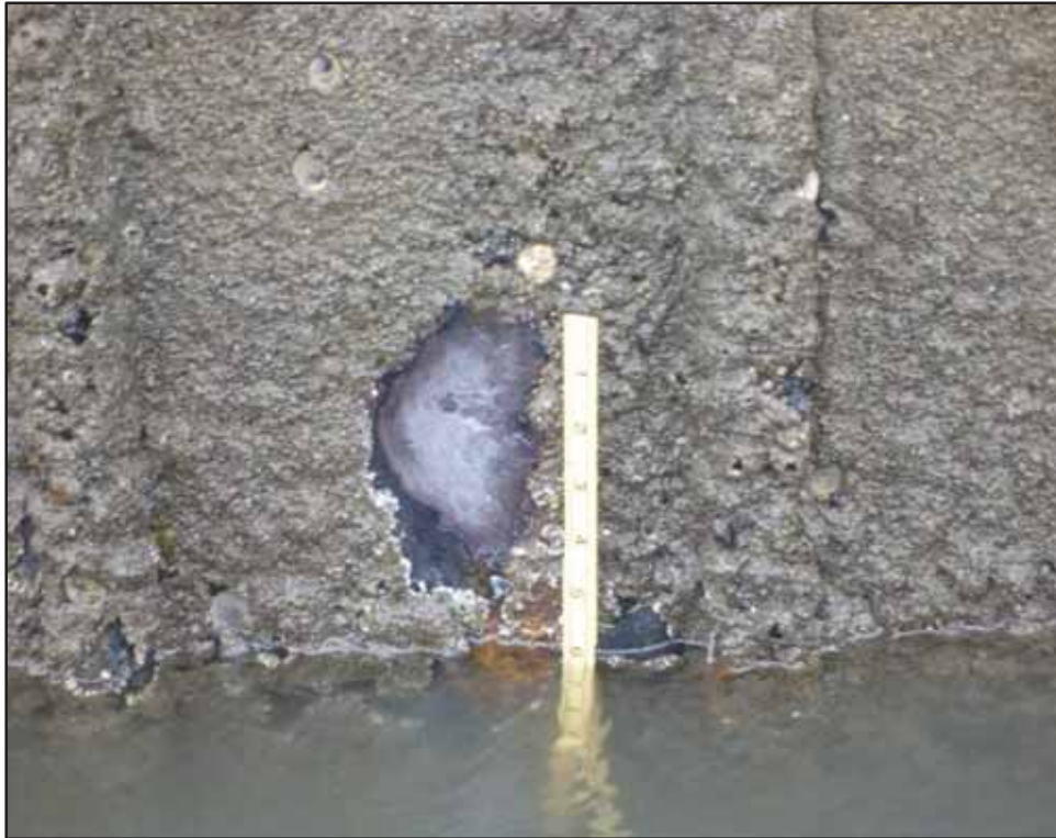
Photo 39-5''H x 3.5''W hole in sheet on west side of bulkhead
