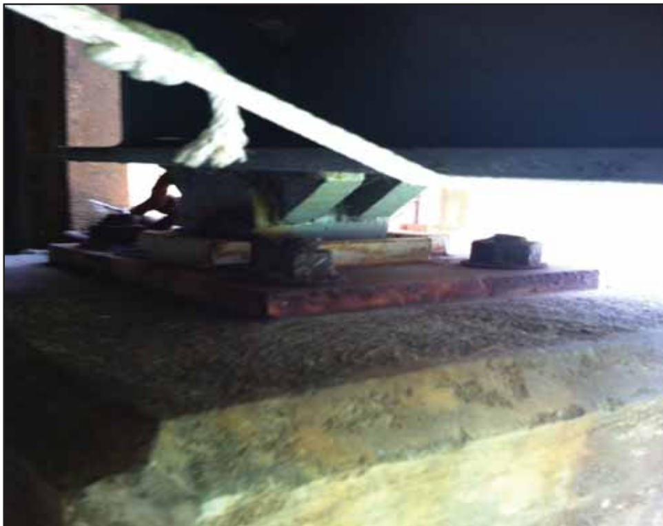
Photo 14-Typical bearing pad corrosion of gangway at Station 7 + 10
