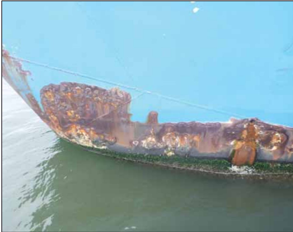
Photo 43-Coating loss in splash zone at Station 0 + 00 on south side of barge
