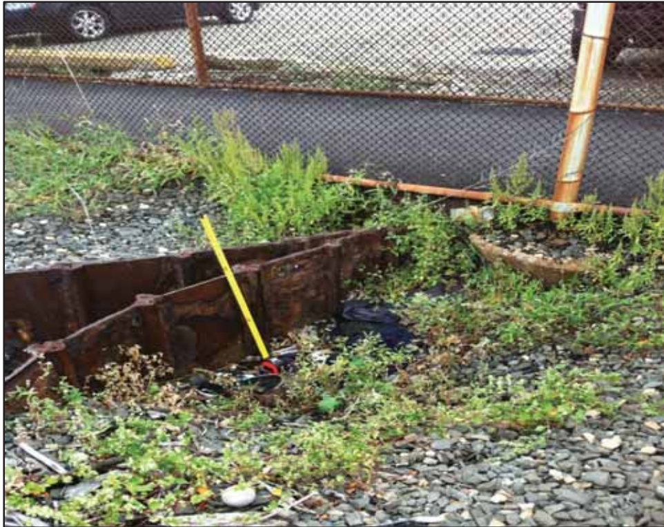
Photo 33-Sinkhole at 1 + 03 7'L x 6'W x 2'D
