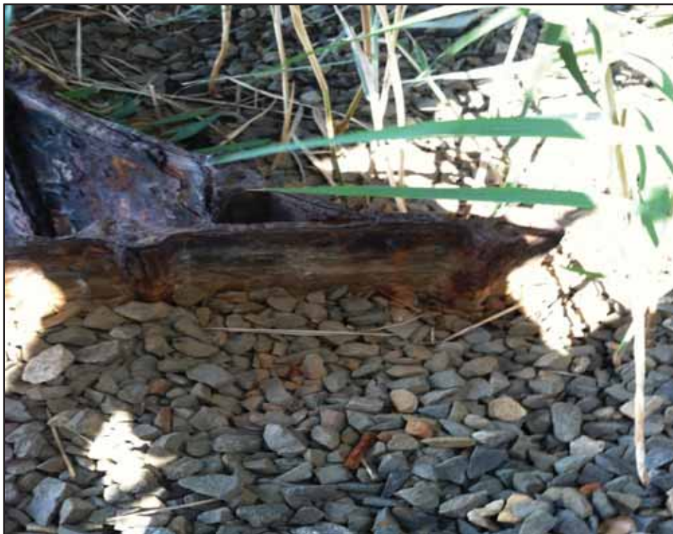
Photo 30-Typical 6in. deep depression at 3 + 05
