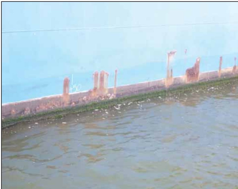
Photo 44-Coating loss in splash zone at Station 1 + 50 on south side
