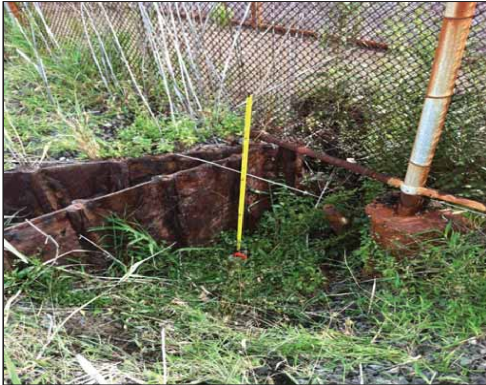
Photo 31-Sinkhole at 0+43 7'L x 11'W x 3'D
