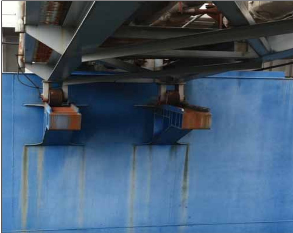
Photo 13-Rollers of utility gangway at Station 6 + 71
