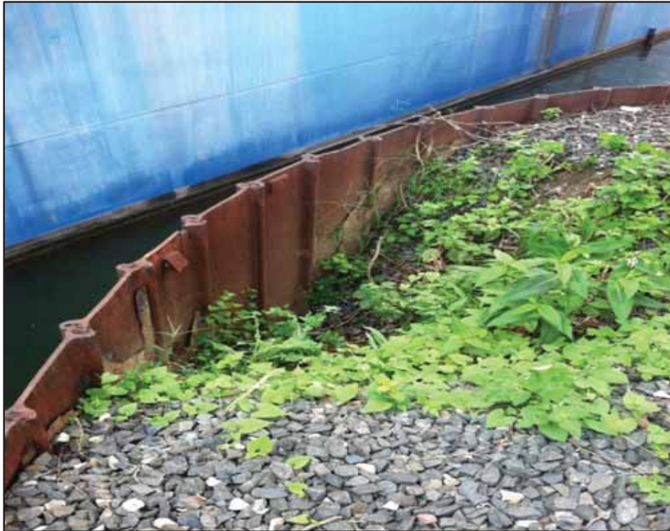
Photo 35-Sinkhole at 7 + 46 10'L x 6'W x 4'D
