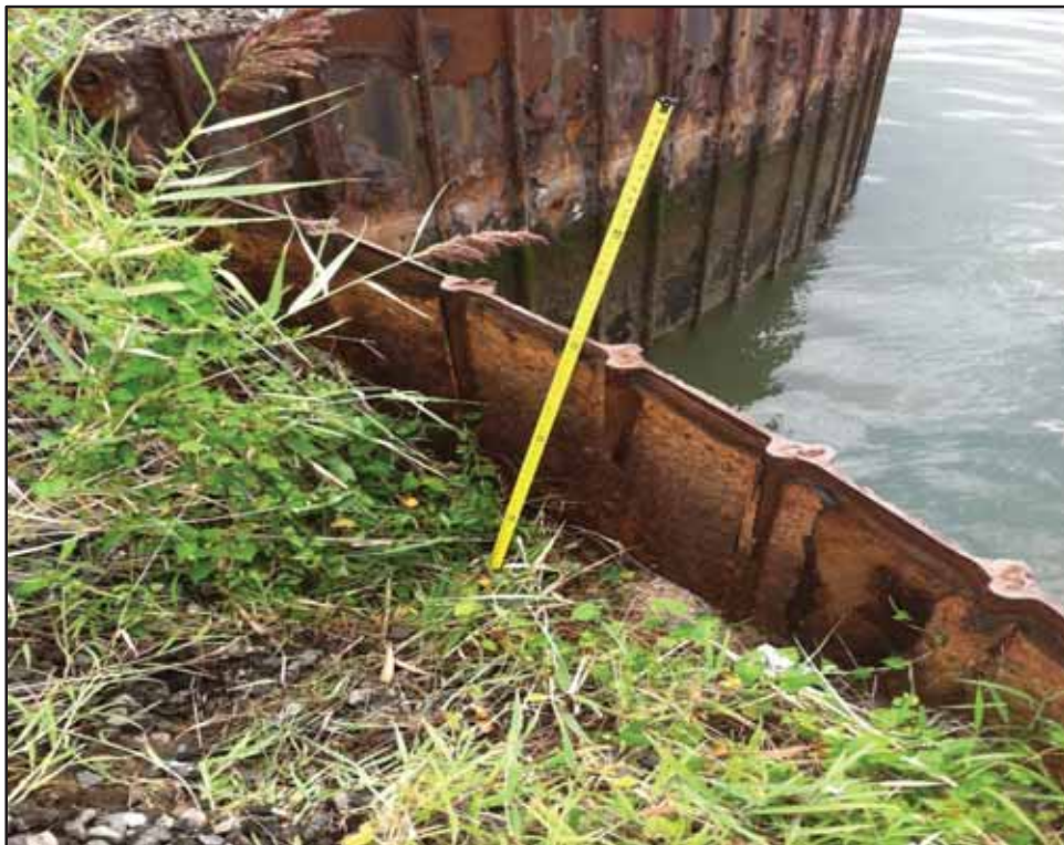
Photo 32-Sinkhole at 0+55 9'L x 7'W x 3'D
