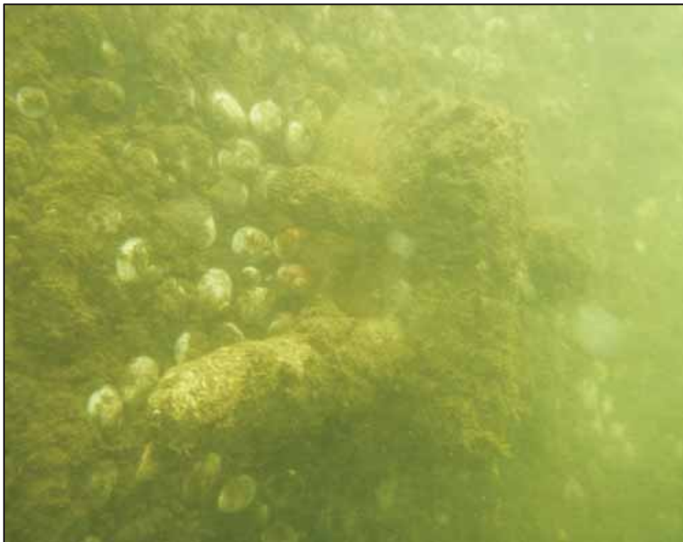
Photo 42-Deteriorated timber bumper at cathodic protection system
