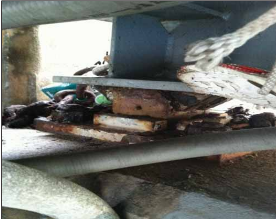
Photo 11-Typical corrosion of landside of gangways at Station 4 + 90
