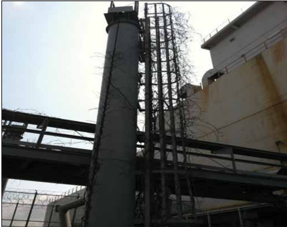
Photo 19-Vine growth on winch tower of utility gangway at Station 7 + 53
