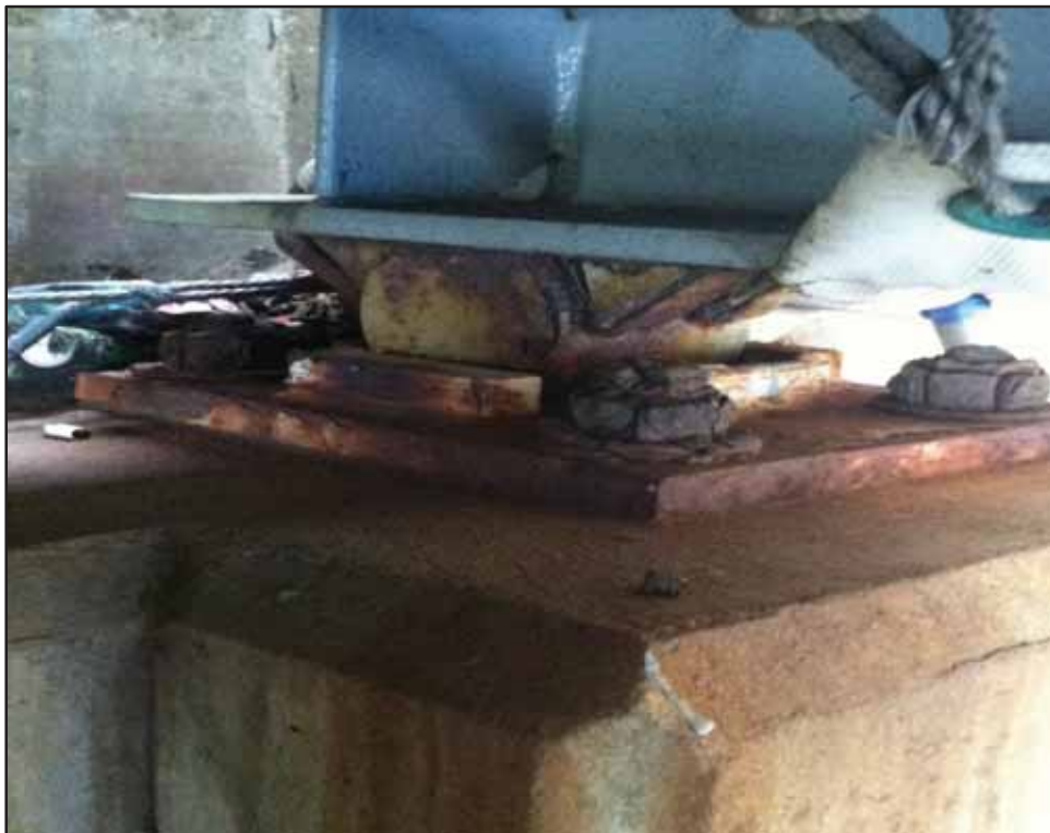
Photo 2-Gangway bearing plate and hardware corrosion at Station 3+10
