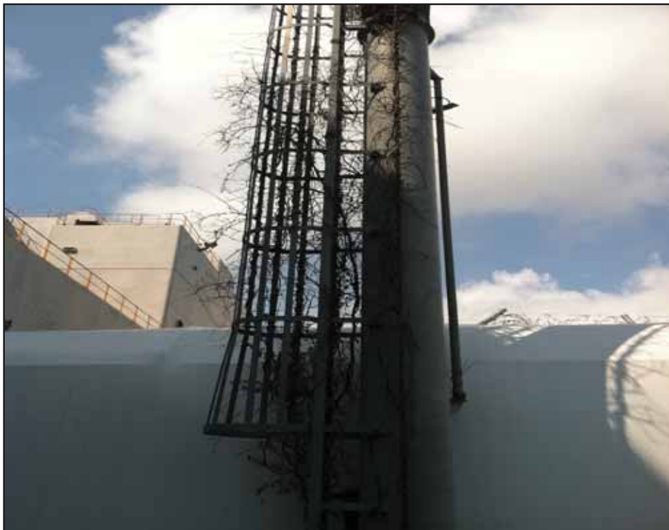
Photo 16-Vine growth on winch tower of gangway at Station 7 + 10
