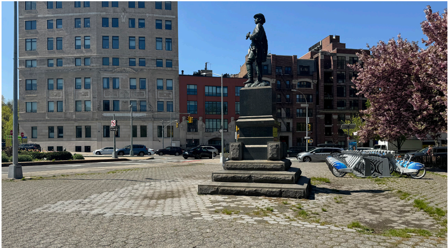
1 - Plaza space around the General Warren sculpture with Bike Sharing Station and paving in poor condition
