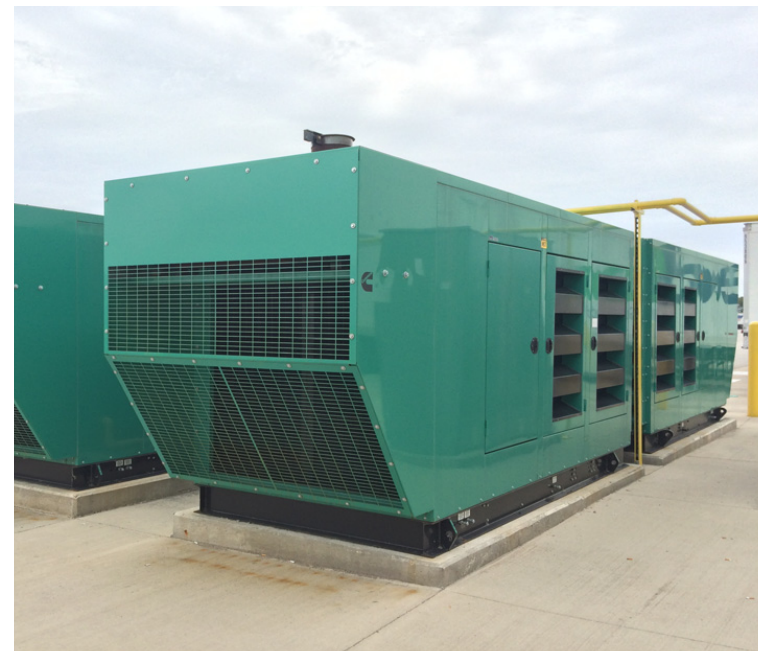
GENERATOR ENCLOSURE LIGHT GRAY METAL COLOR
