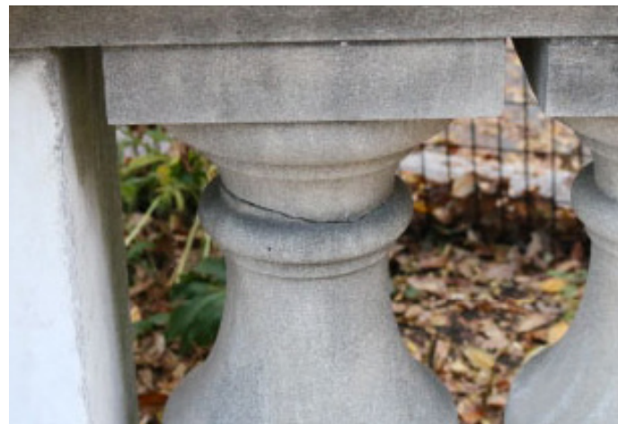
Full Unit Limestone Crack
