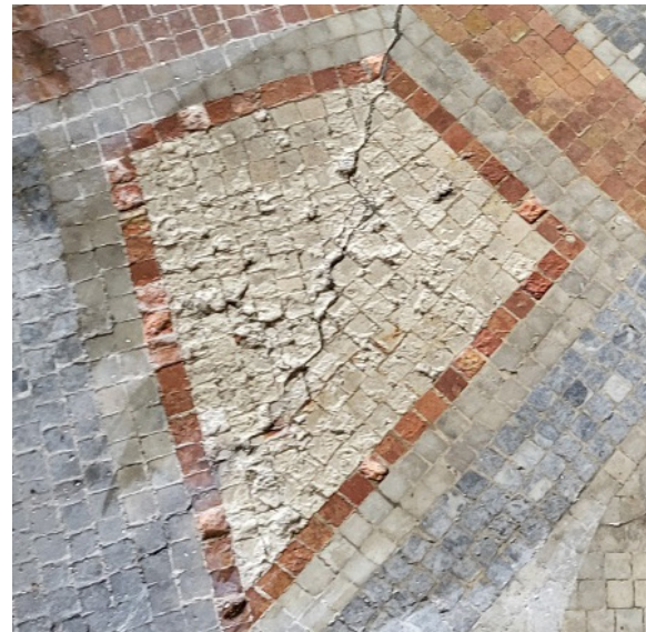
Floor Crack and Material Lost
