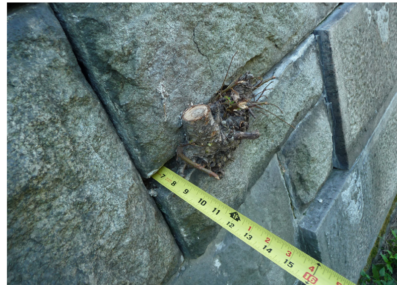
Biological Growth and Displacement
