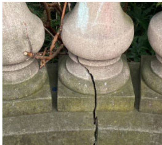
Full Unit Limestone Crack
