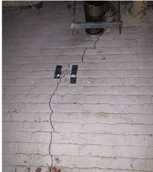
Photo 1 – Cellar – North Foundation Wall – Vertical Crack below the Pipe with Crack Gage #2
