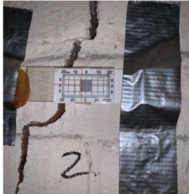
Photo 2 – Cellar – North Foundation Wall – Vertical Crack below Pipe with Enlarge Crack Gage #2
