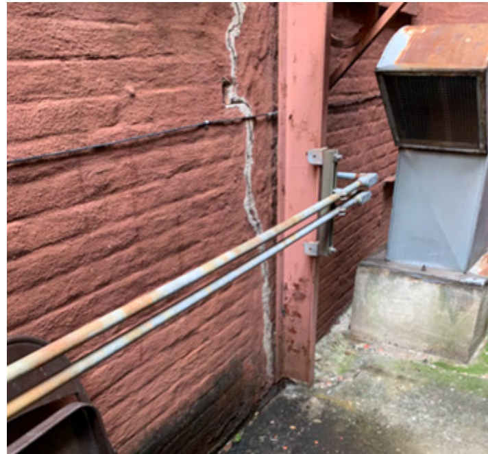
Photo 3 – West Elevation – Crack at the Apparatus Floor Window Overall View
