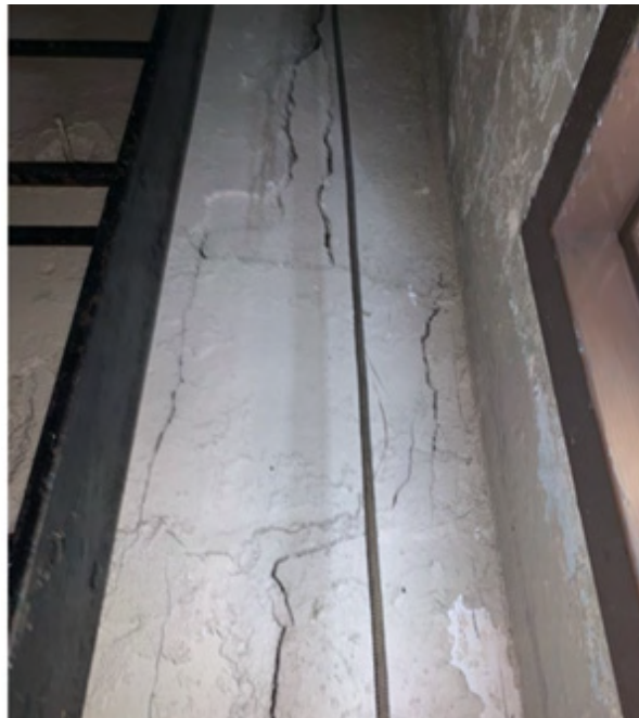
Photo 5 –North Side Hose Tower - Vertical Crack at the Interior
