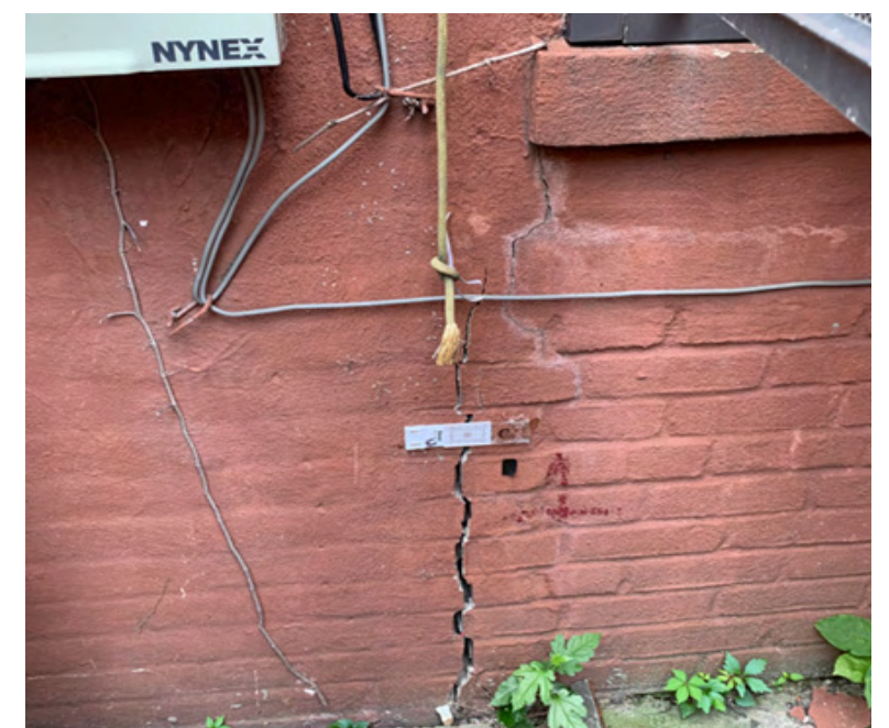
Photo 8 – West Elevation – Diagonal Cracks below the Kitchen Window (See Crack Gage on Photo 9)
