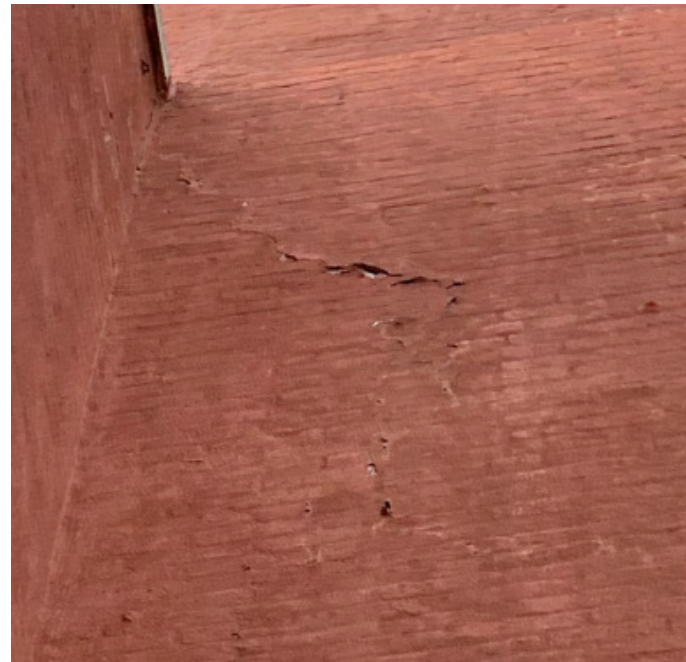
Photo 6 –North Side of the Hose Tower -Diagonal Cracks at the Exterior
