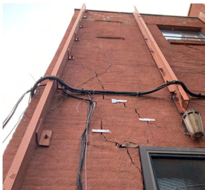
Photo 7 – West Elevation – Diagonal Cracks above the Kitchen Window
