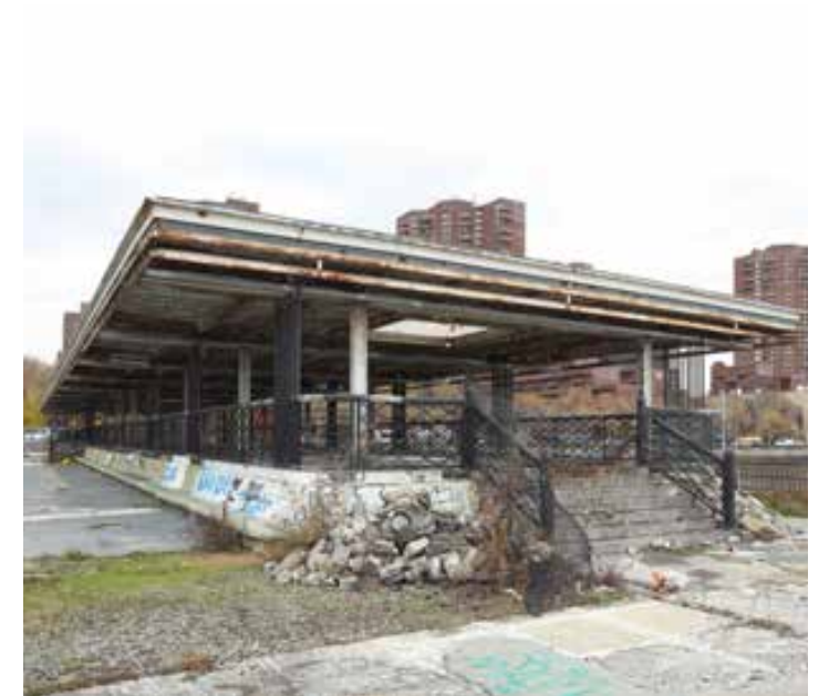
2018 Pier closed to the public due to structural deterioration
