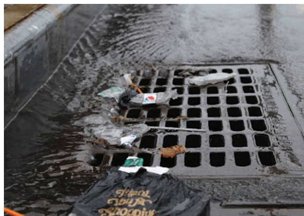
Debris on a storm drain.
