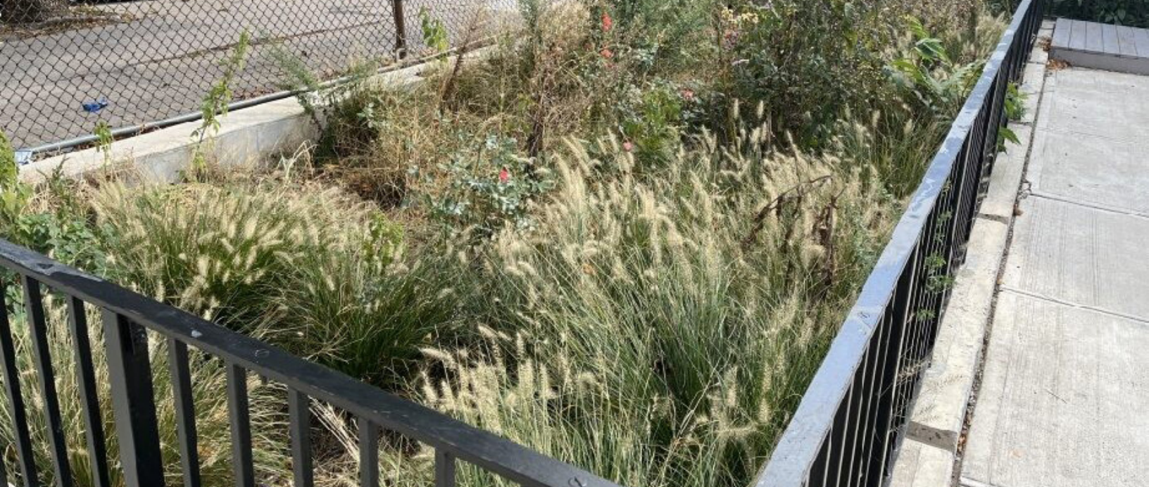
A completed bioretention practice at K238: Anne Sullivan in the Coney Island Creek MS4 area.
