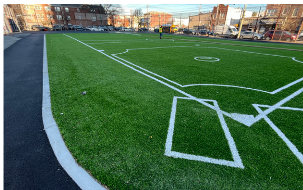
Completed synthetic turf practice with subsurface stone storage at KO95: Gravesend in the Coney Island Creek MS4 area.
