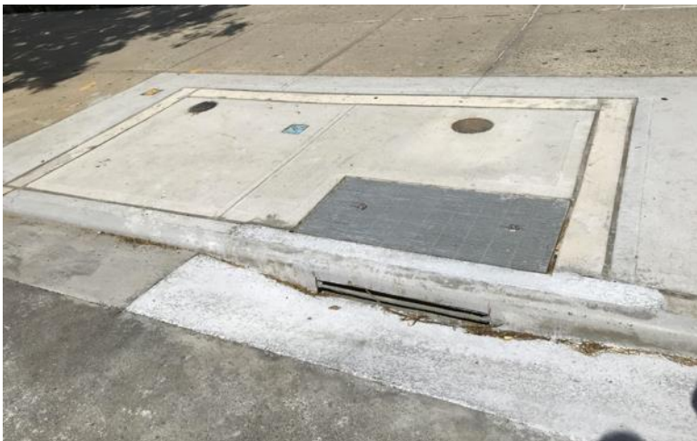
Left : Infiltration Basin with Concrete Top Right : Infiltration Basin with Grass Top
